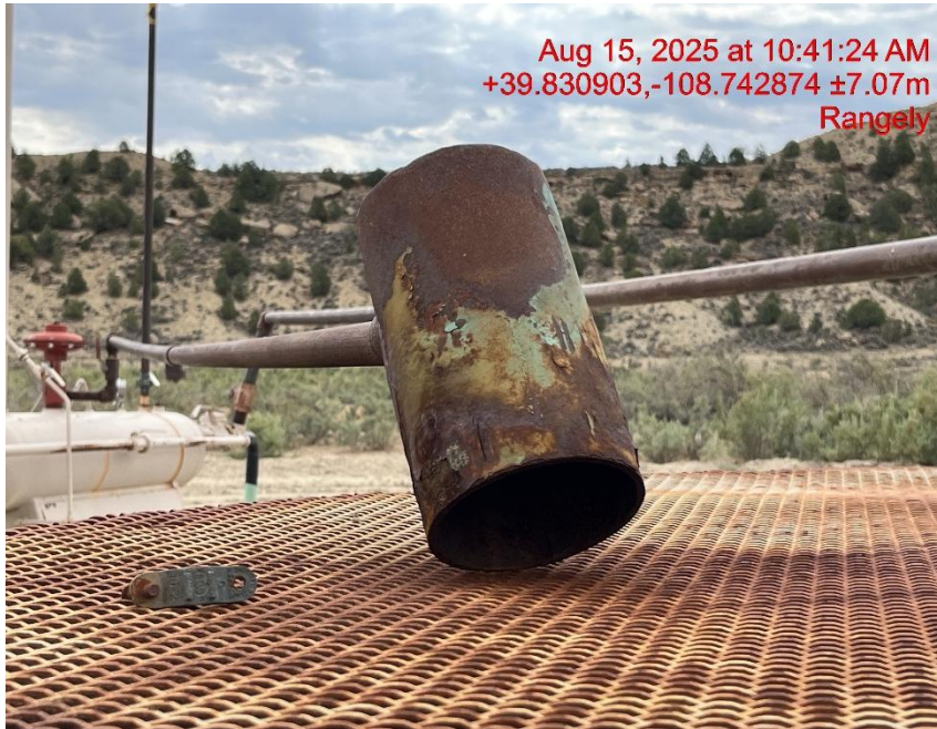
Photo # 1979 Open ended piping/wildlife hazard/available for entry by wildlife
