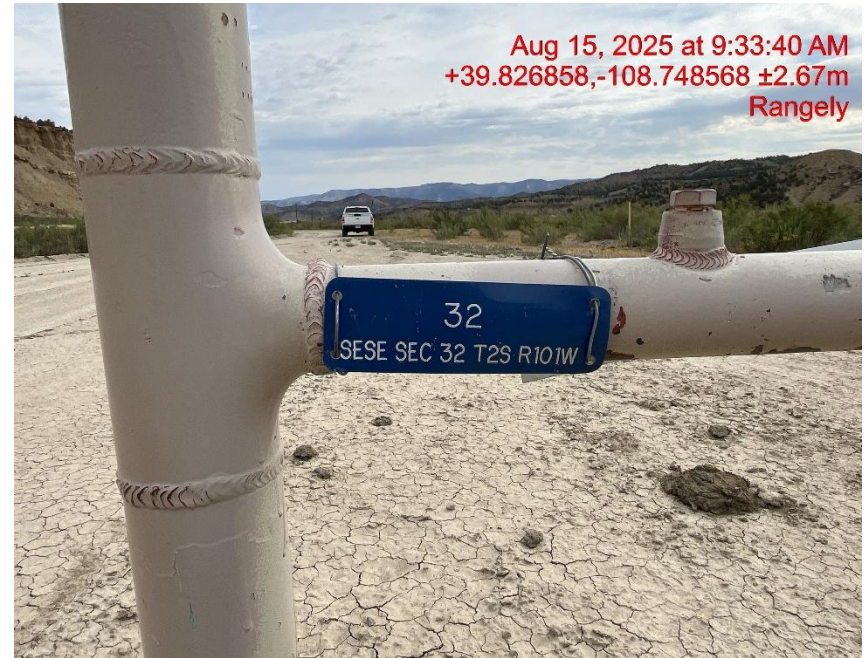
Photo # 1922 Wellhead sign lacks required information
