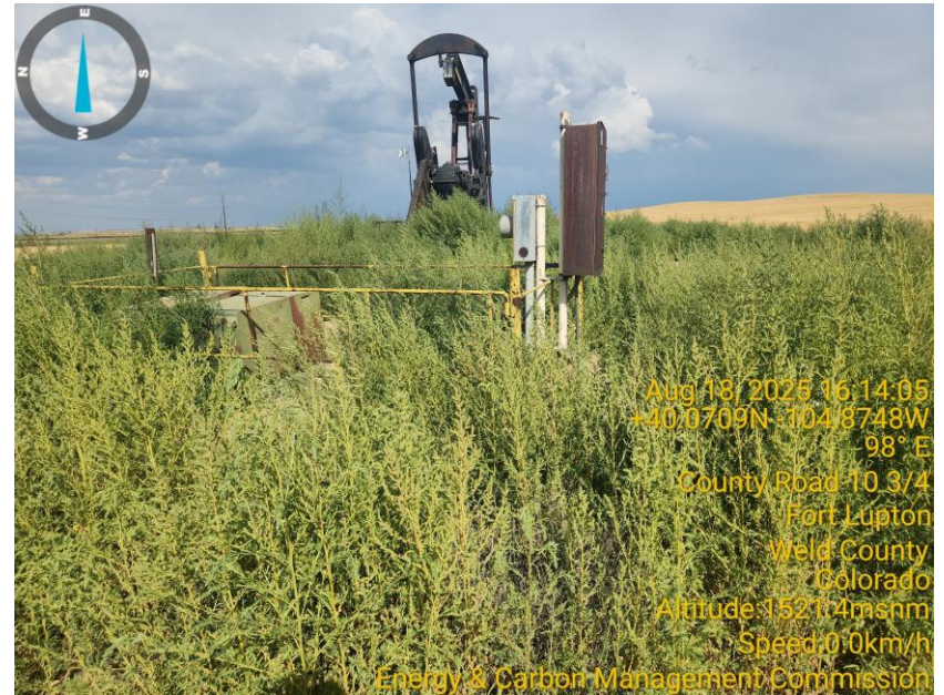
Photo 2 Ancillary equipment overrun with tall vegetation.
