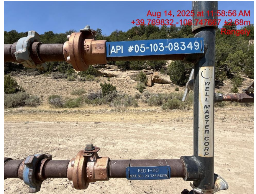
Photo # 1848 Wellhead sign lacks required information
