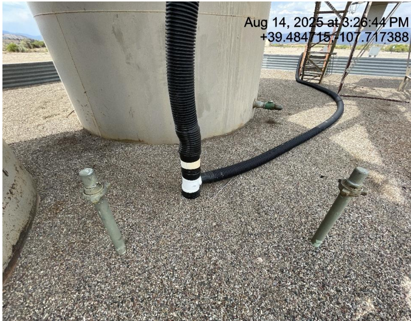
Photo # 953 Unused flowlines lack lockout tagout (OOSLAT)
