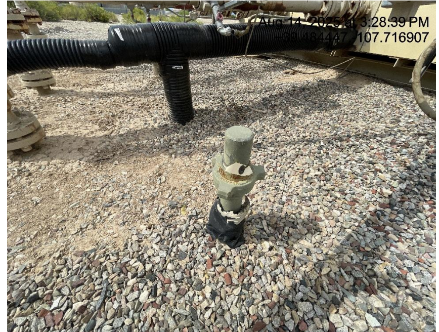
Photo # 952 Unused flowline lacks lockout tagout (OOSLAT)
