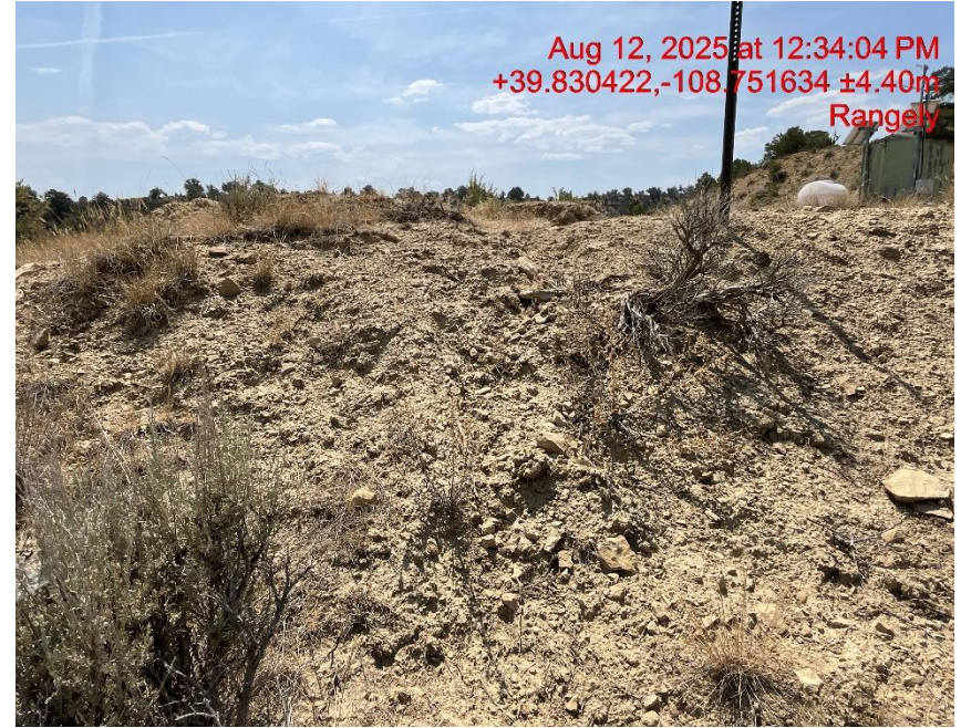
Photo # 1803 Failure to minimize erosion & transport of sediment off location/insufficient BMP's
