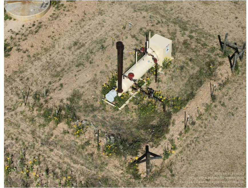
Location/ Overgrown Vegetation
