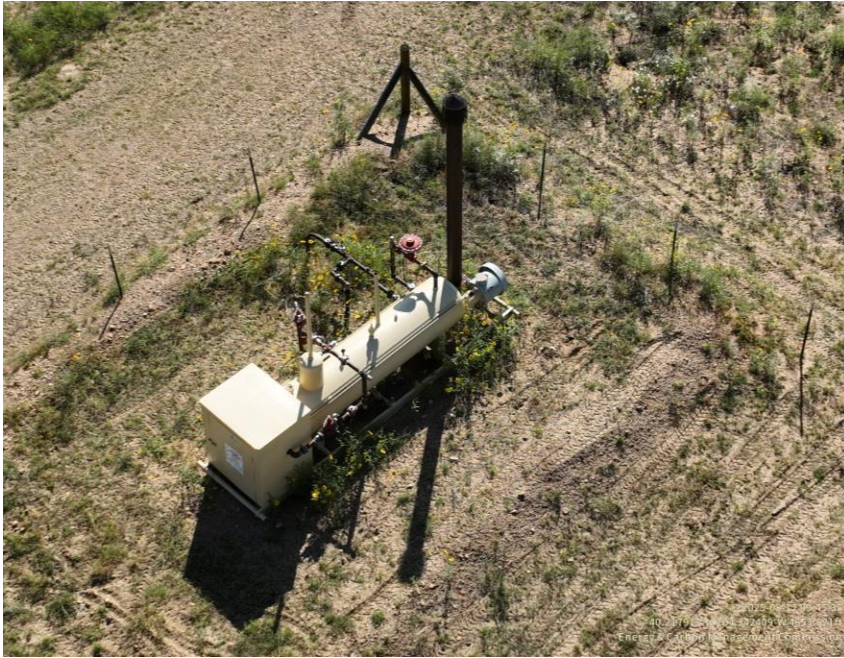
Location/ Overgrown Vegetation
