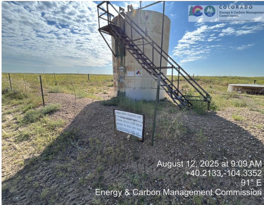
Production Tank/ Overgrown Vegetation
