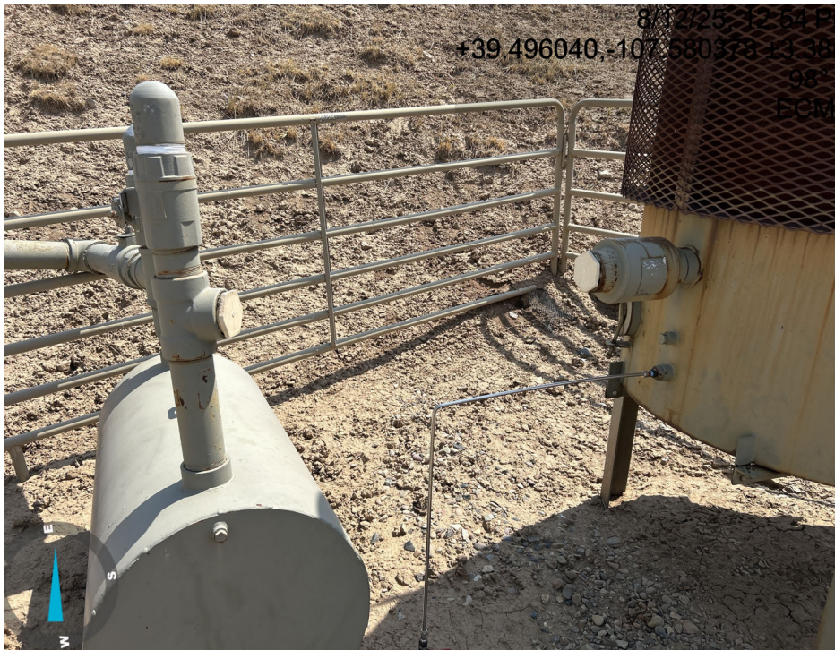
Line to ECD from tanks not connected to ECD
