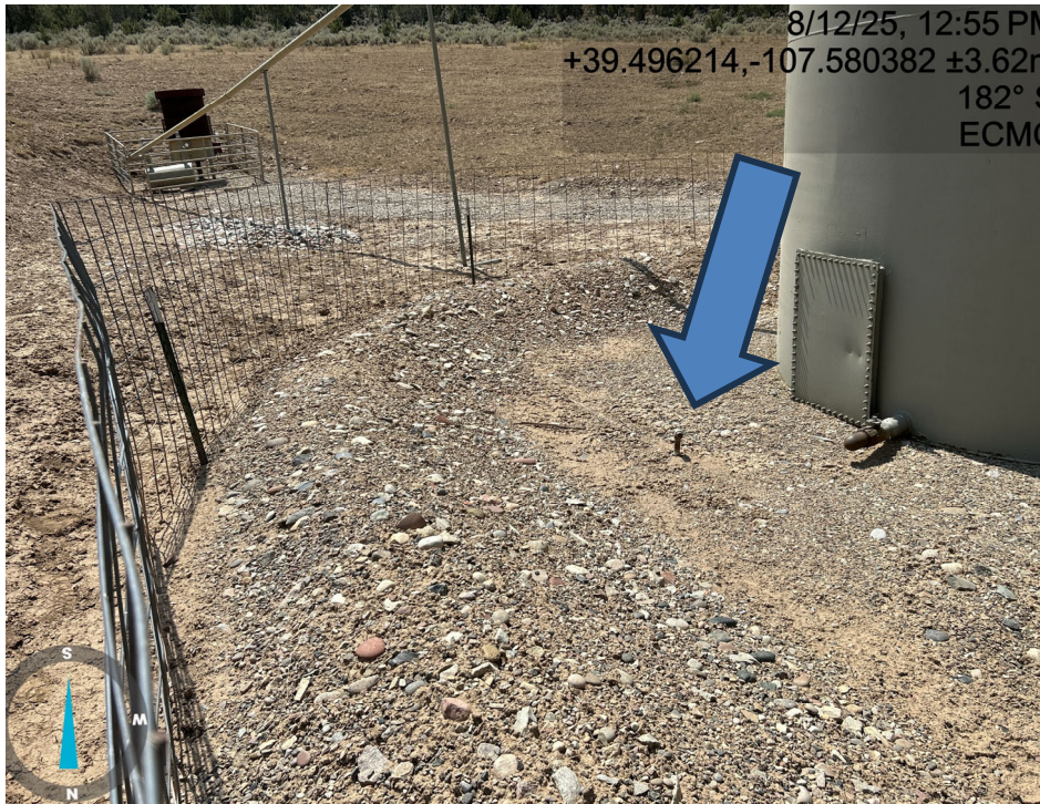
Capped and disconnected supply gas line to ECD
