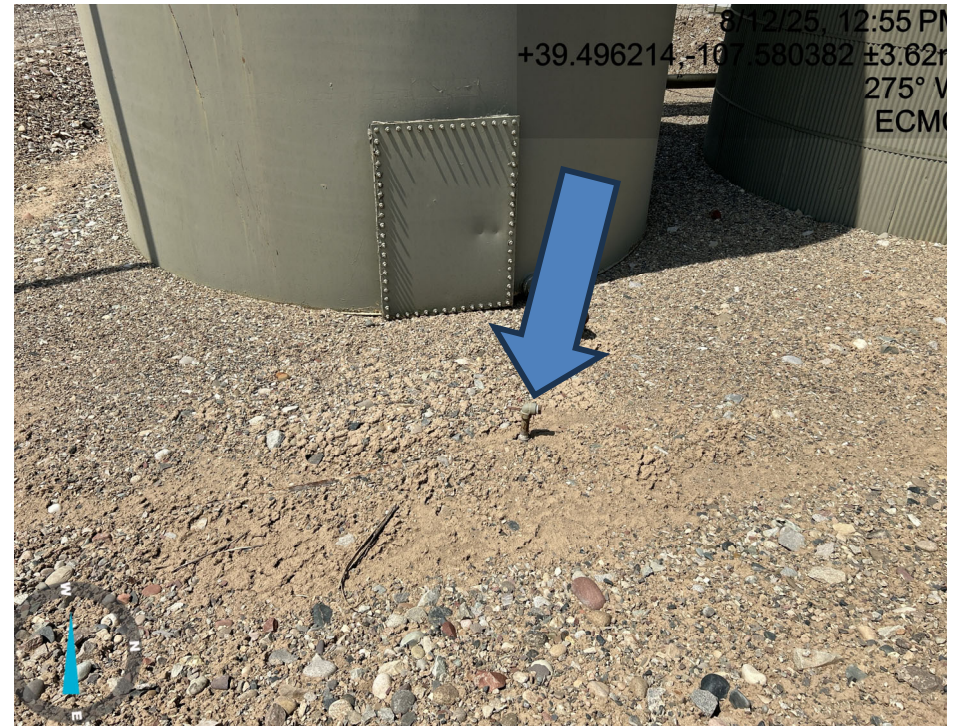
Capped and disconnected supply gas line to ECD
