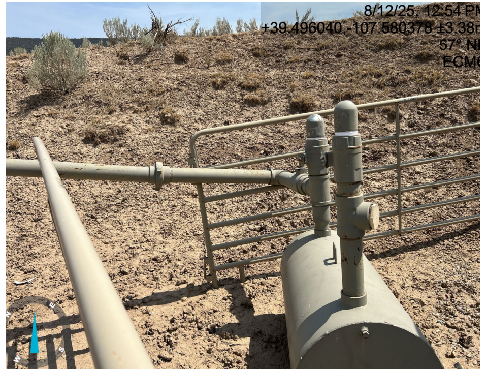
Line to ECD from tanks not metered
