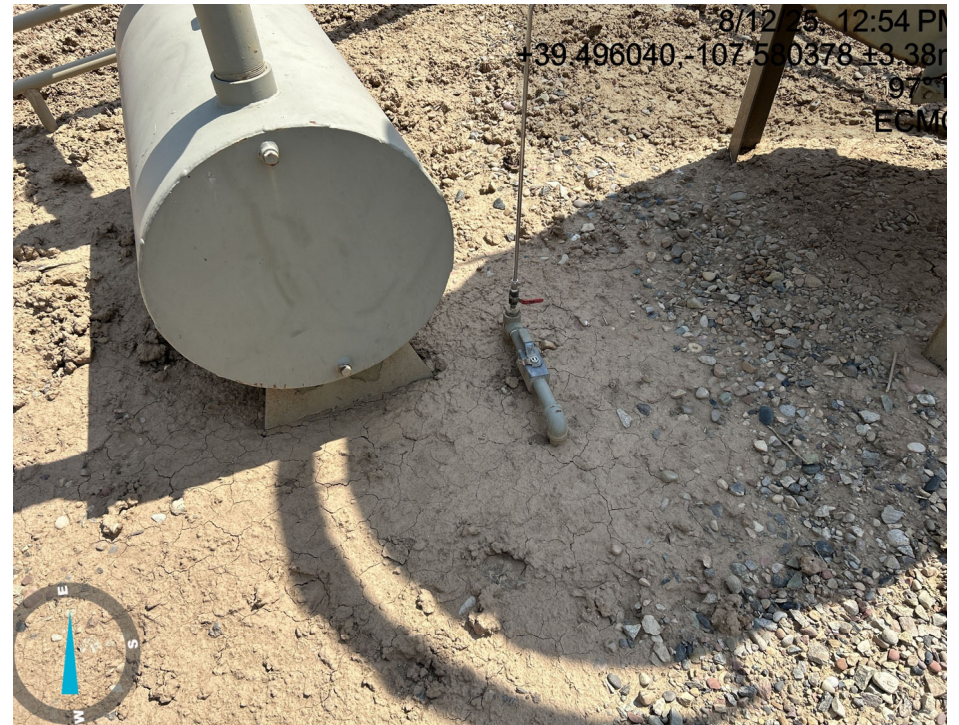
Supply gas line for pilot is connected to ECD and shut. Other end if 1 inch line is disconnected at tank battery
