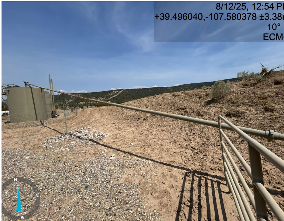
Line to ECD from tanks not metered
