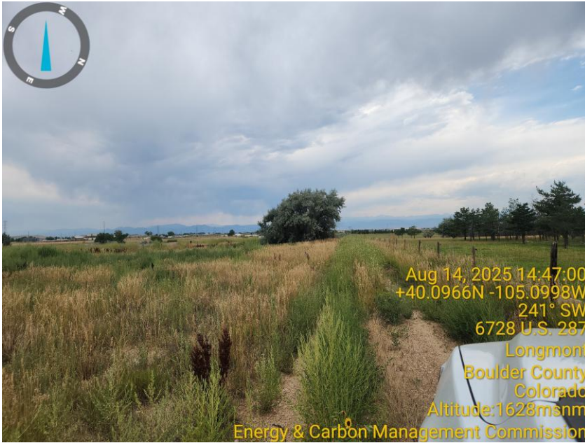
Photo 1 Access road overrun with tall vegetation.
