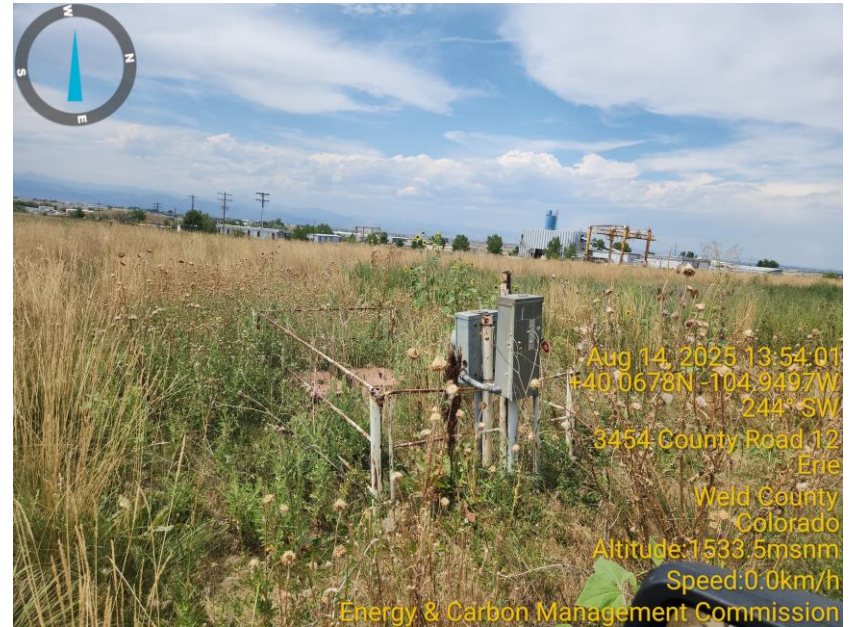
Photo 4 Ancillary equipment overrun with tall vegetation
