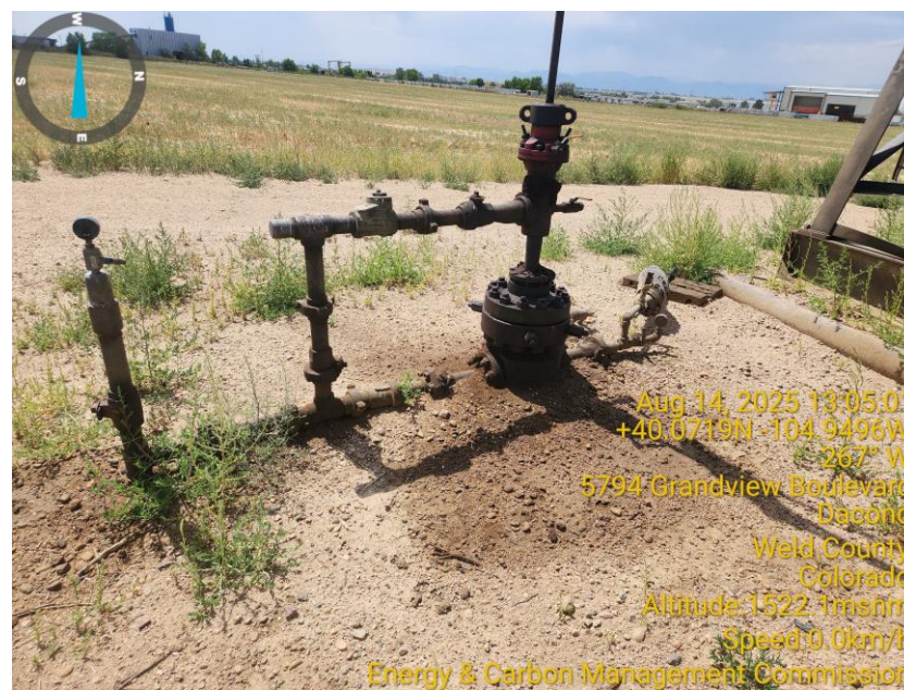
Photo 2 Stained soil around the Wellhead.
