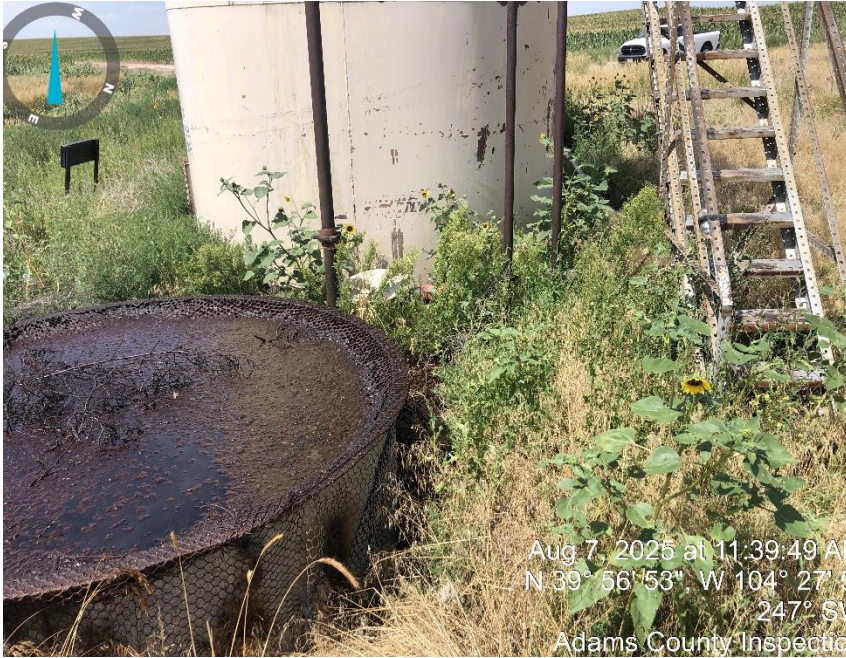
Photo #5 Open top tank flowing over.
