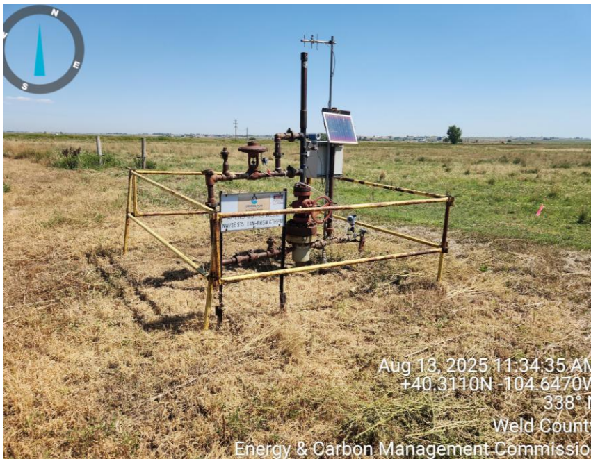
Photo 1 well head and equipment
