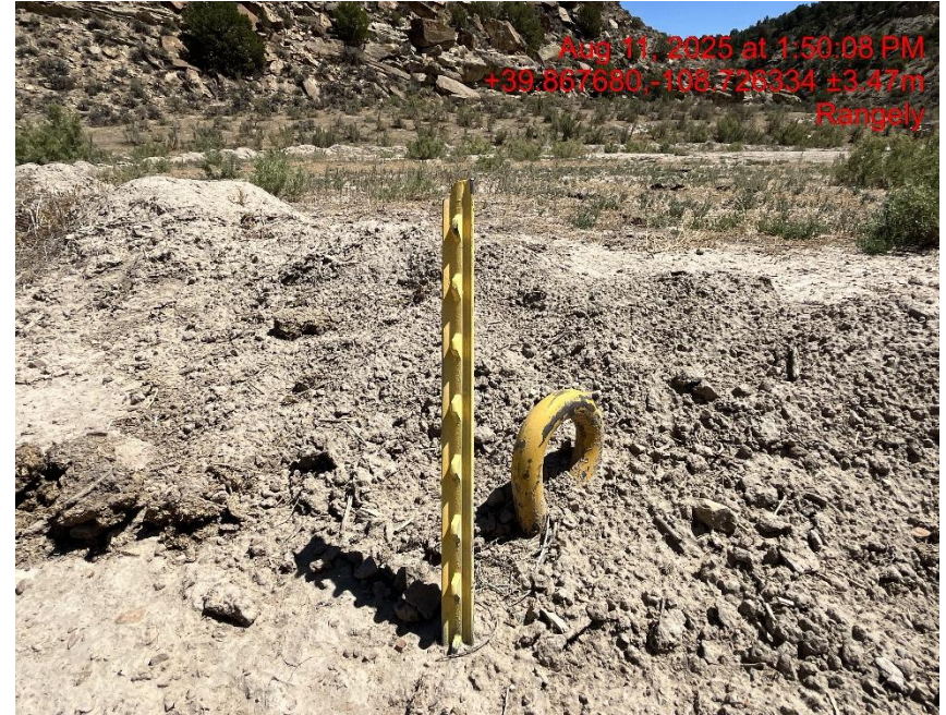
Photo # 1723 Improperly marked deadman
