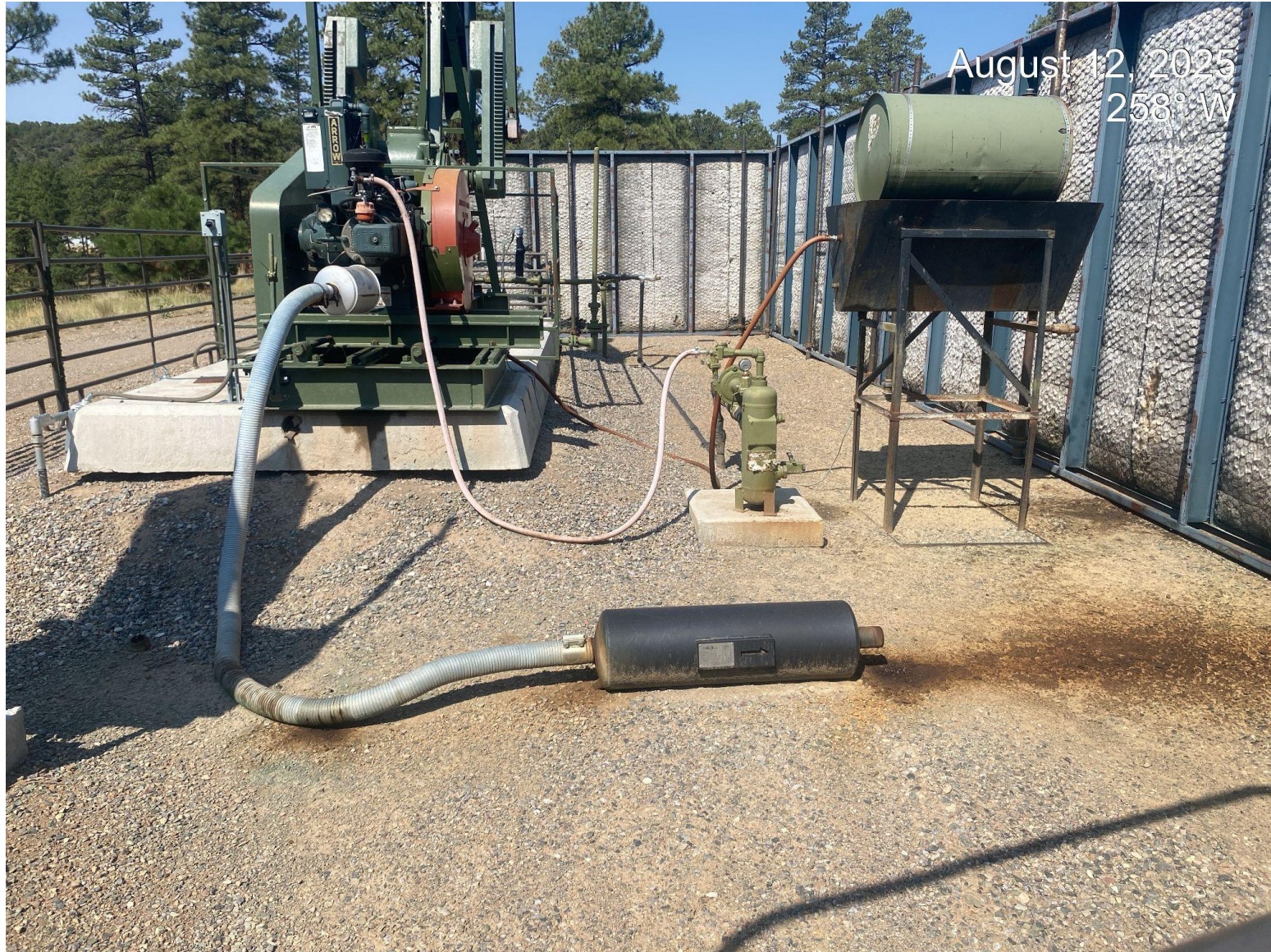
Photo 2. Stained soils at pump jack muffer.
