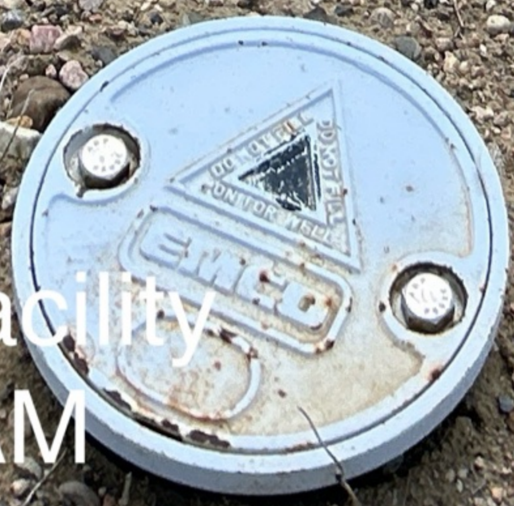
Looking east-southeast at the monitoring and remedial well network. A flush mount well is visible in the foreground; PVC stickup wells are visible in the background.
