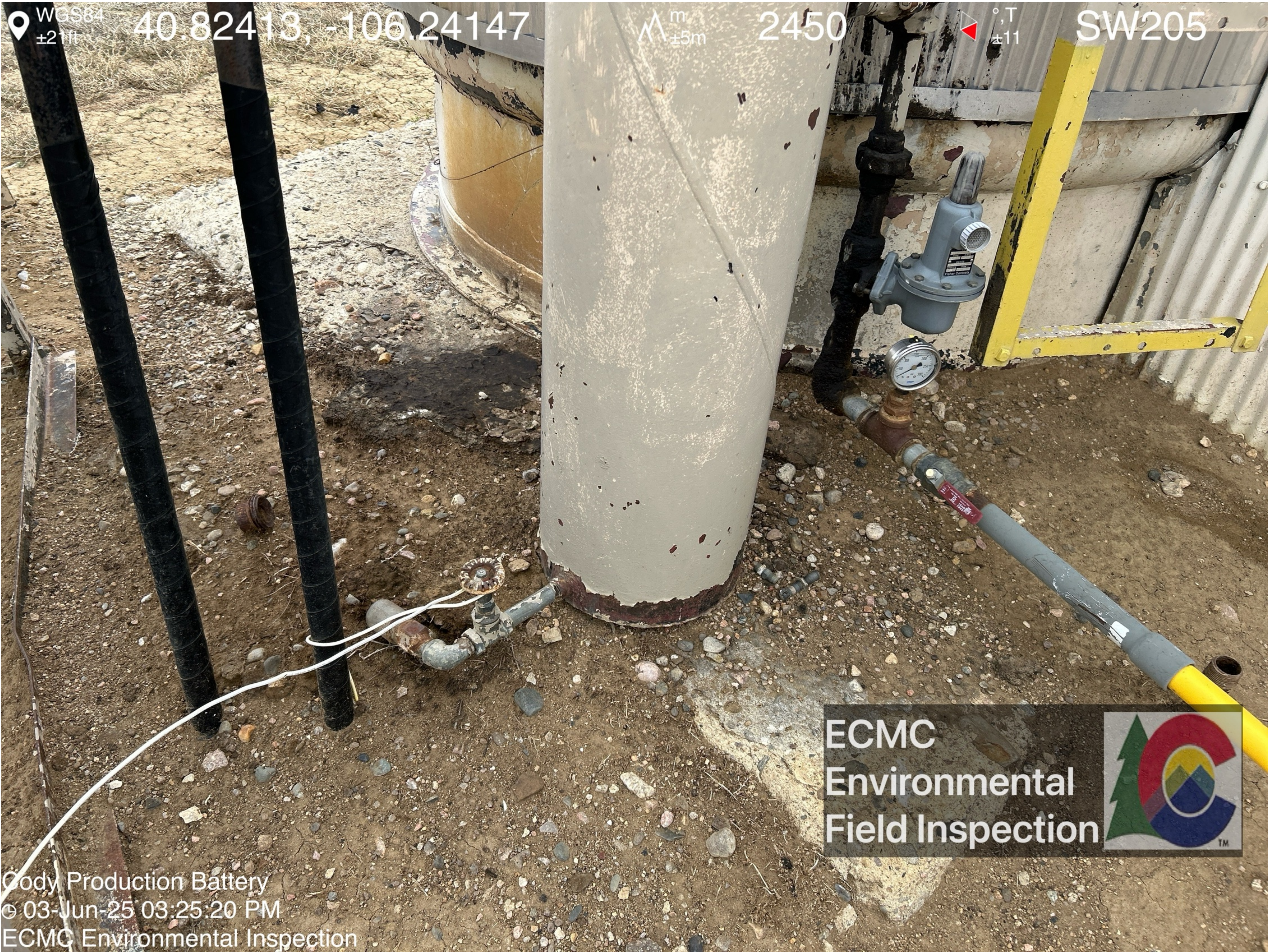
Stained soil is visible adjacent to the separator. A strong petroleum hydrocarbon odor was observed when the stained soil was disturbed.
