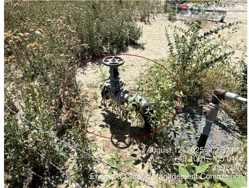
Unmarked Risers/ Overgrown vegetation
