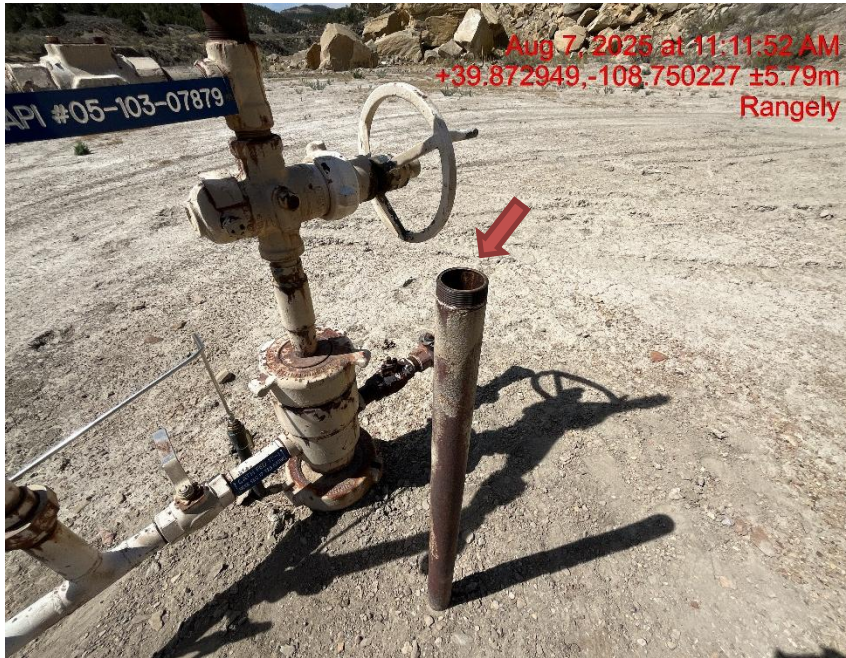
Photo # 1500 Open ended piping/wildlife hazard/available for entry by wildlife
