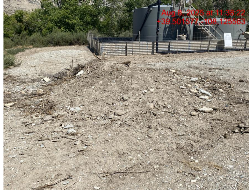
Soil Stockpile on Location with no BMPs Installed – Photo #00085
