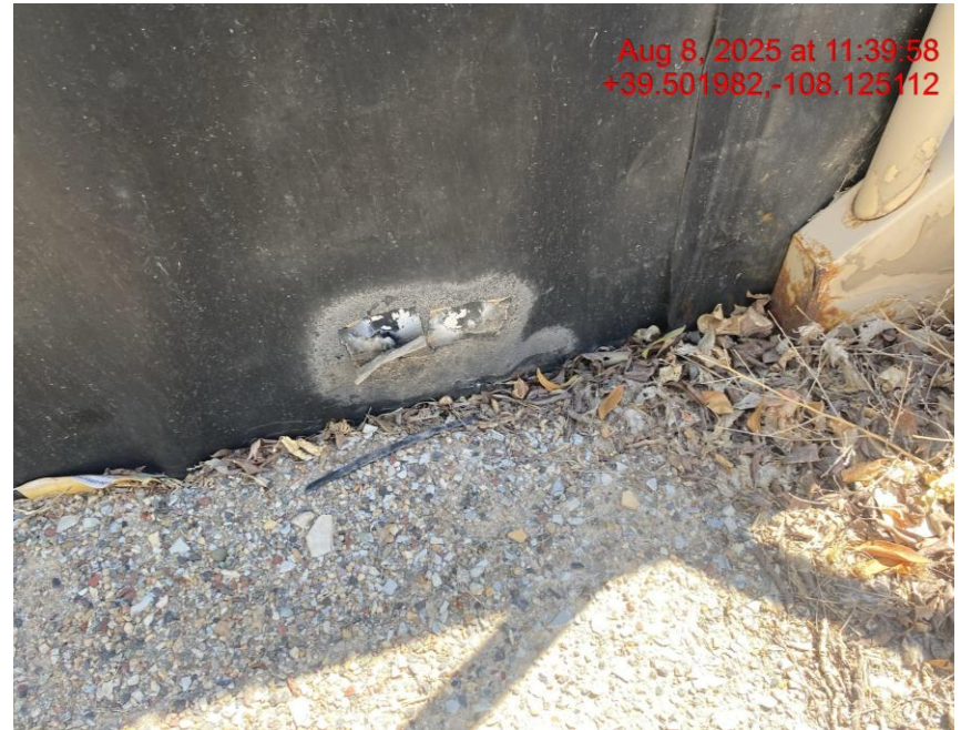
Hole in Containment Liner – Photo #00089
