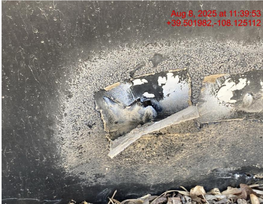
Hole in Containment Liner – Photo #00088
