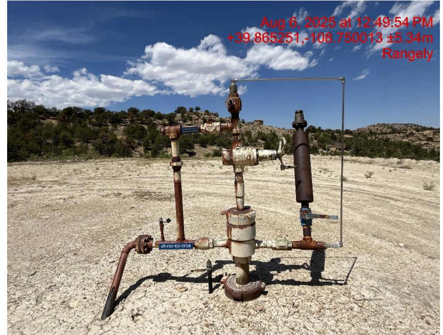
Photo # 1454 Wellhead sign lacks required information
