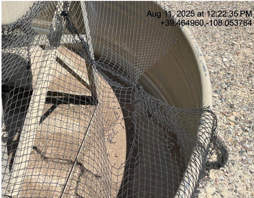
Photo # 9649 Wildlife protection needs maintenance /wildlife hazard
