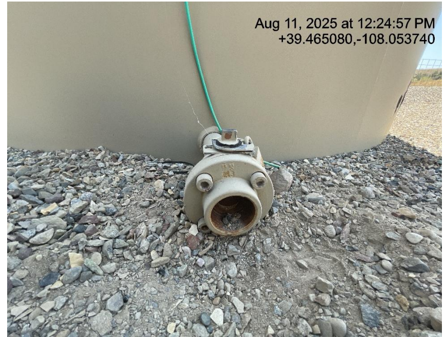
Photo # 9648 Open ended load line
