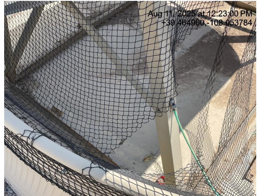
Photo # 9650 Wildlife protection needs maintenance /wildlife hazard
