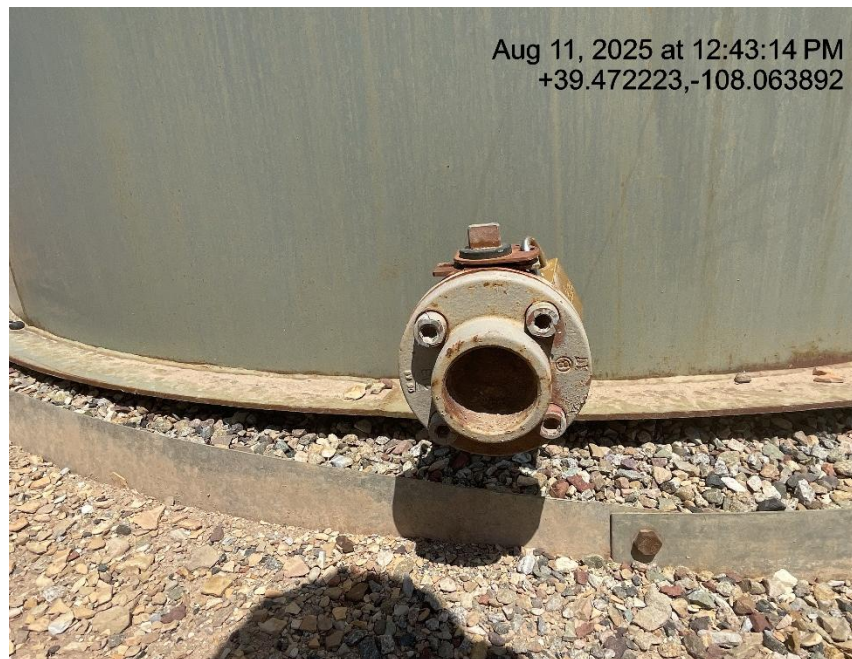
Photo # 9704 Open ended load line
