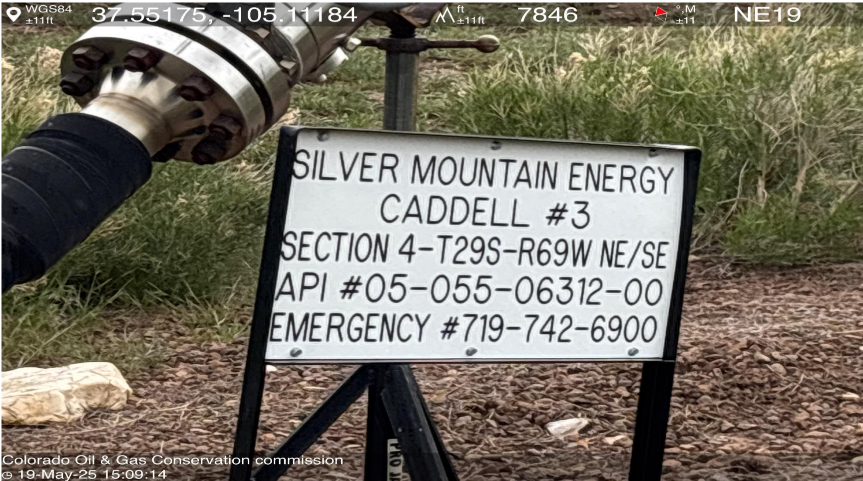
PHOTO 3: CURRENT OPERATOR IS NOT LISTED ON WELL SIGN/ API # IS NOT ACCURATE. ECMC RECORDS SHOW CADDELL #3 API # IS 05-055-06319 AND 911 IS NOT INCLUDED AS AN EMERGENCY CONTACT ON WELL SIGN. Install sign to comply with Rule 605.e. CA DATE 8-22-2025
