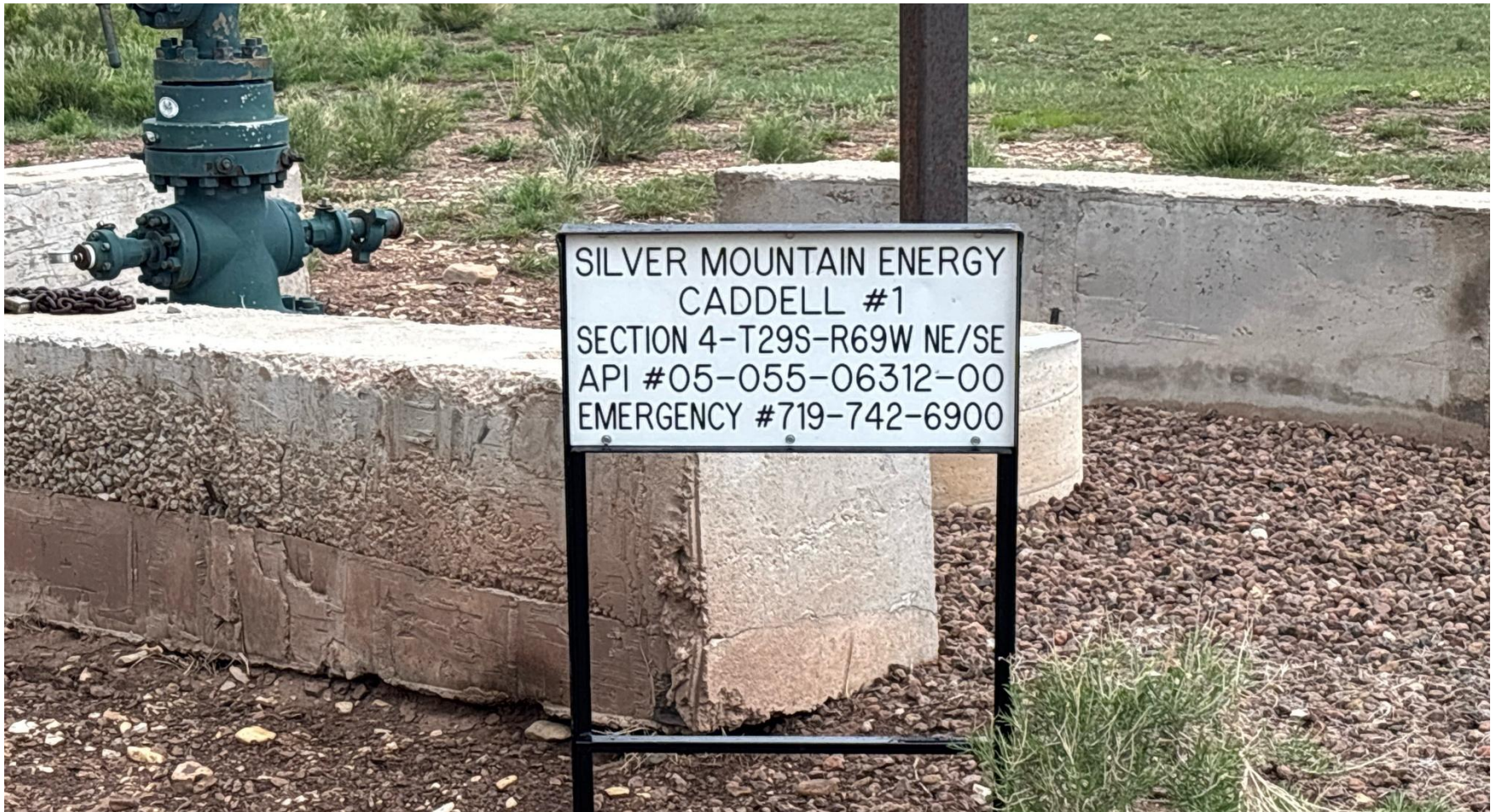
PHOTO 1: CURRENT OPERATOR IS NOT LISTED ON WELL SIGN/ API # IS NOT ACCURATE ECMC RECORDS SHOW CADDELL #1 API # IS 05-055-06285 AND 911 IS NOT INCLUDED AS AN EMERGENCY CONTACT ON WELL SIGN. Install sign to comply with Rule 605.e. CA DATE 8-22-2025.
