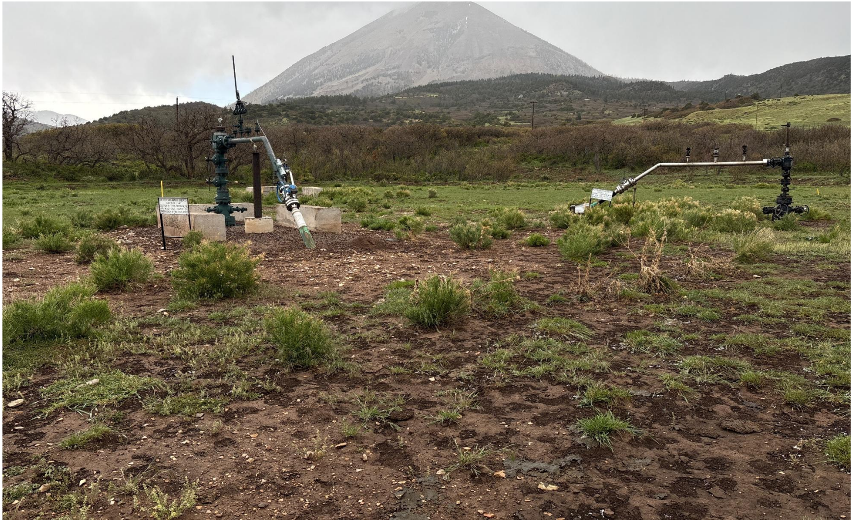
PHOTO 8: TALL SHRUBS AROUND LOCATION. MAINTAIN WEEDS PER RULE 606. 8-22-2025
