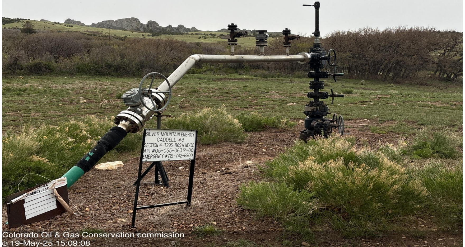
PHOTO 6: WELLHEAD AND EQUIPMENT.
