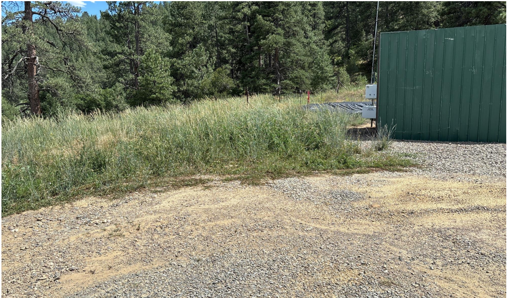
PHOTO 4: WEEDS ARE ENCROACHING ON WELLHEAD EQUIPMENT. MAINTAIN WEEDS PER RULE 606. CA DATE 8-16-2025.
