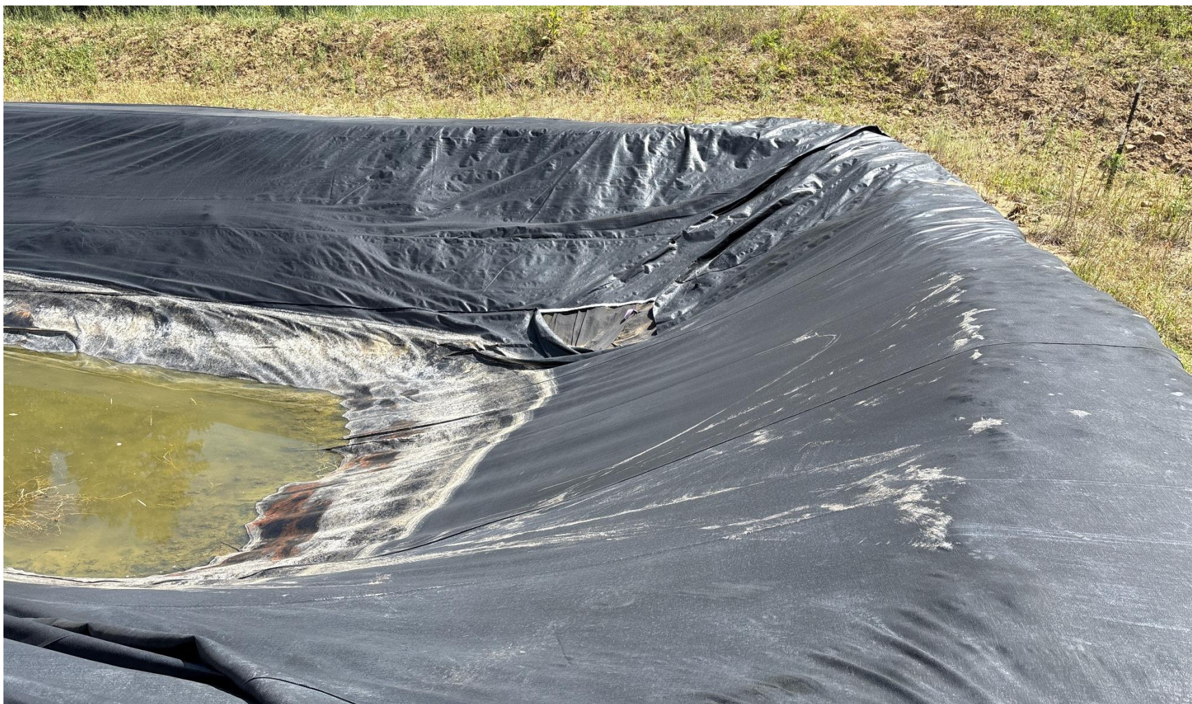
PHOTO 7: PRODUCE WATER PIT LINER IS COMPROMISED. REPAIR LINER OR (Rule 910) Reduce fluid level in pit, contact ECOM EPS staff for directives. THIS IS THE SECOND NOTICE FOR THIS CORRECTIVE ACTION IMMEDIATE ACTION IS REQUIRED.
