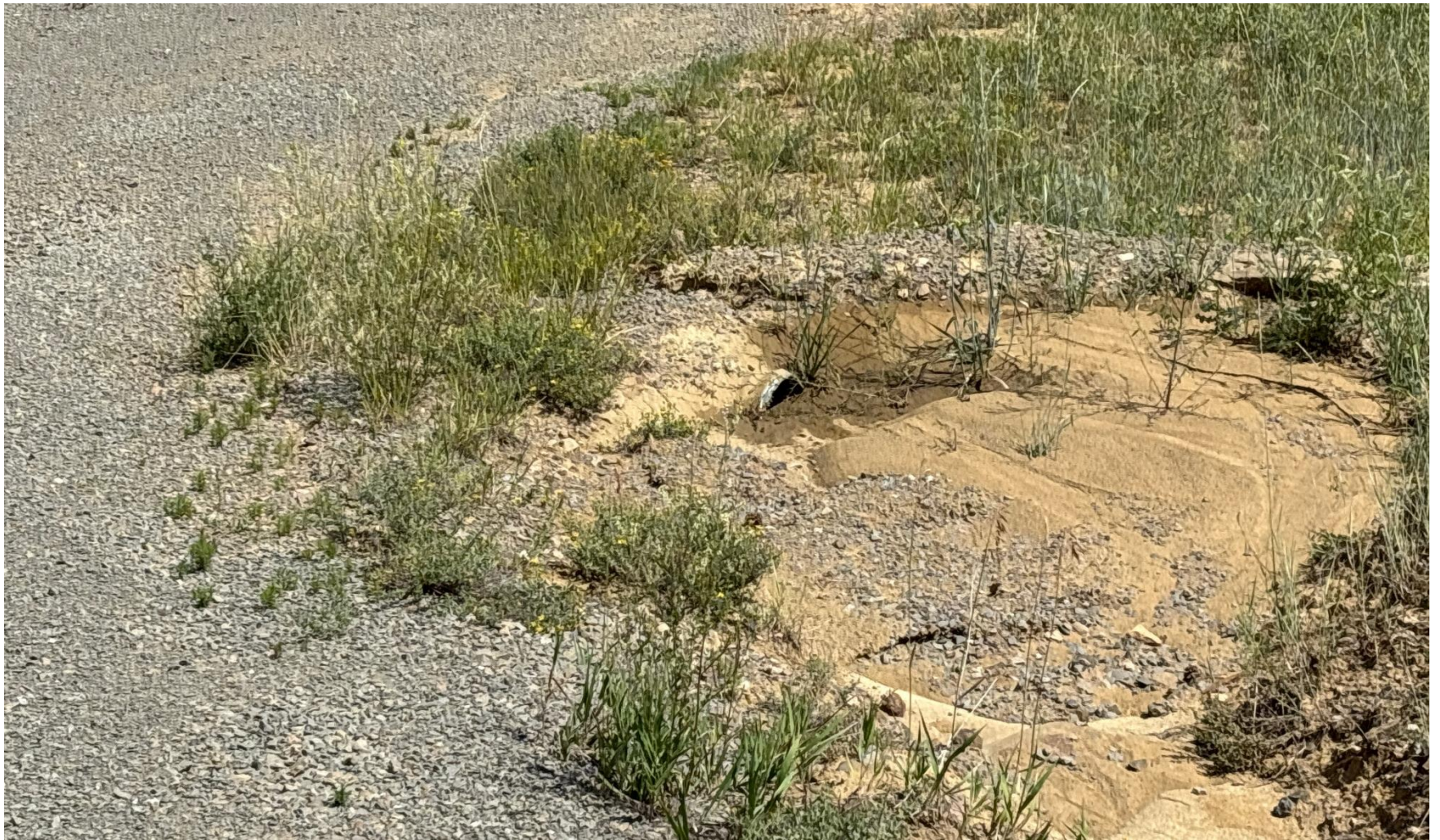
PHOTO 5: CULVERT IS PLUGGED. Install or repair required BMPs per Rule 1002.f.(2)C . CA DATE 6/13/2025.
