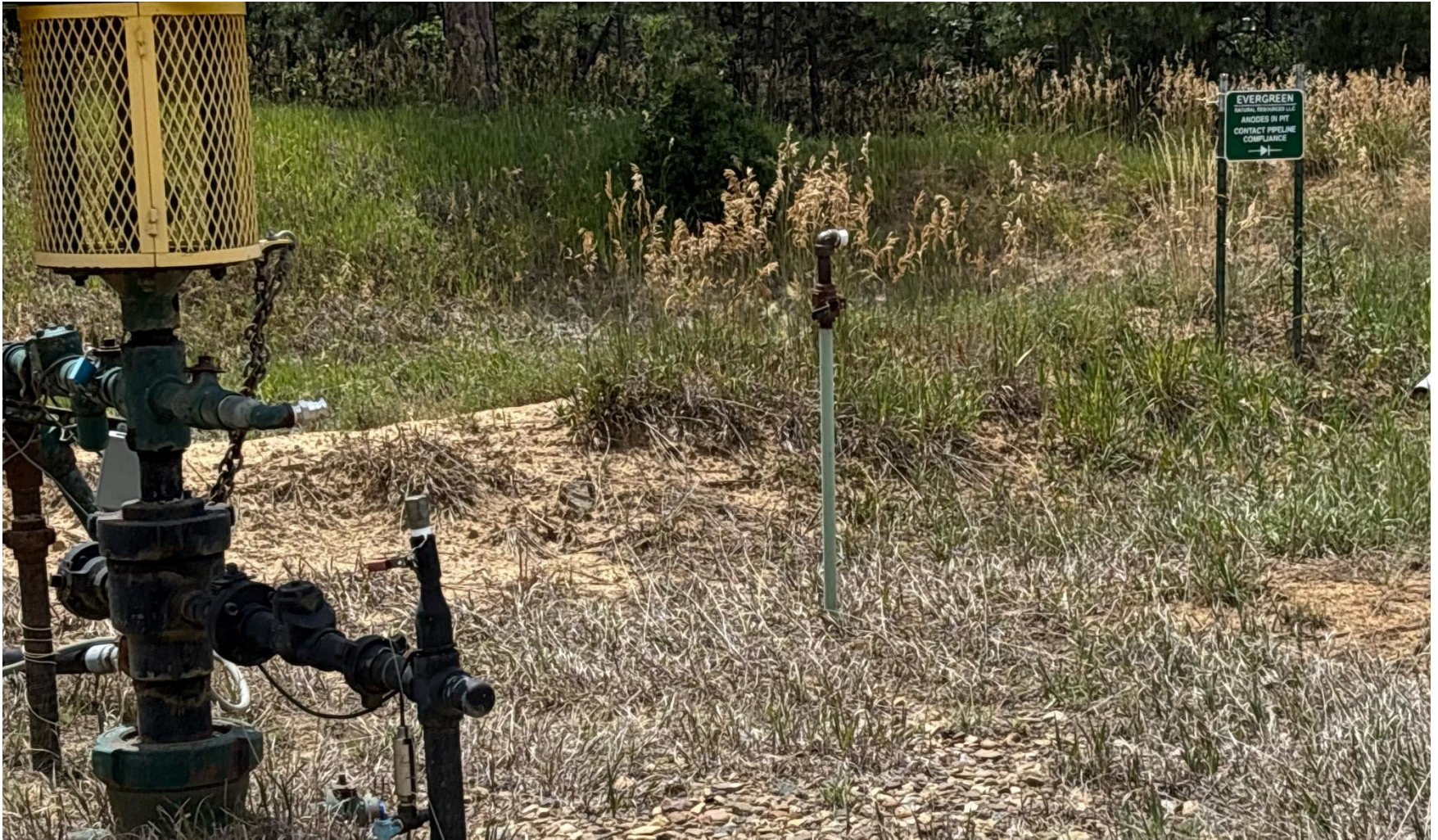
PHOTO 8: UNUSED EQUIPMENT (1" RISER NOT MARKED OR IN USE). REMOVE OR MARK RISER AS TO WHAT IS CARRIES ie. Gas water etc per rule 606. THIS IS THE SECOND NOTICE FOR THIS CORRECTIVE ACTION IMMEDIATE ACTION IS REQUIRED.
