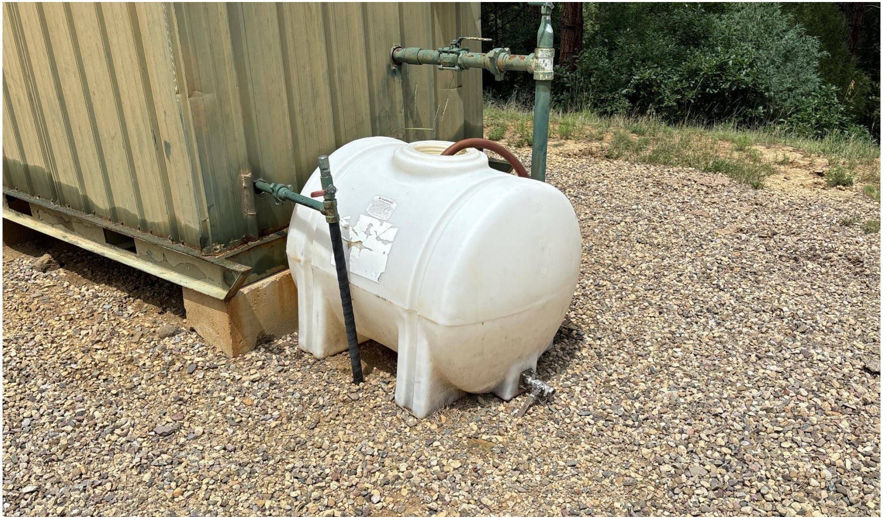
PHOTO 5: PRODUCED WATER DRIP TANK HAS NO LID/ NO WILDLIFE PROTECTION. Install or repair wildlife protection equipment. CA DATE 8-22-2025.
