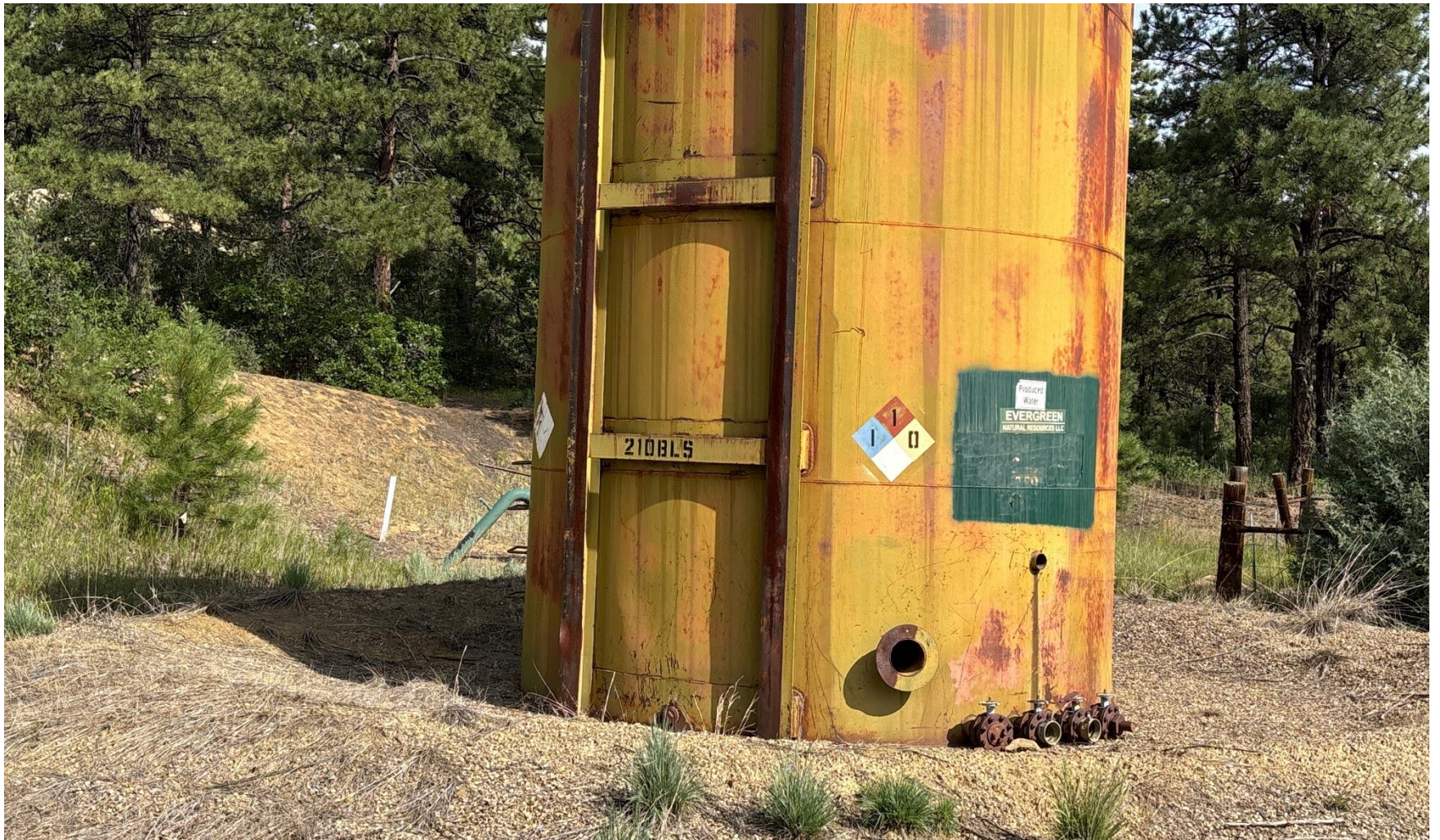
PHOTO 4: PRODUCED WATER TANK BATTERY.
