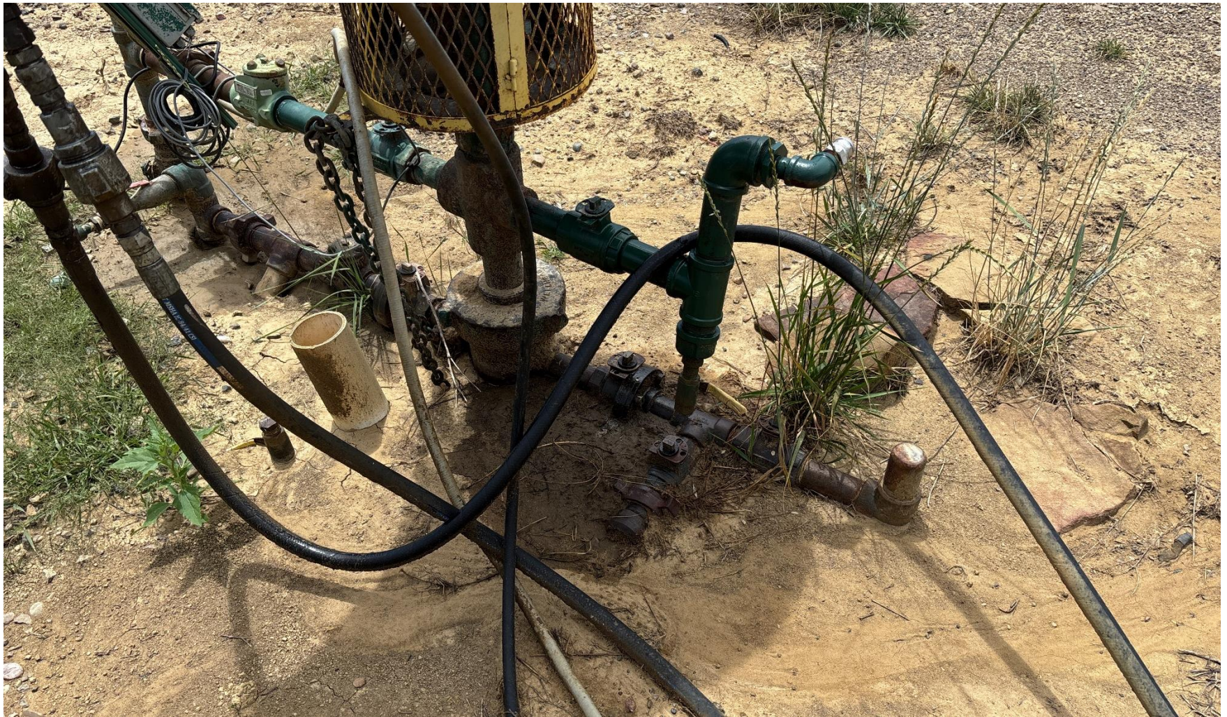
PHOTO 4: PHOTO 5: AREA OF IMPACTED SOIL AROUND WELLHEAD APPEARS TO BE LEAKING HYDRAULIC HOSES AND DRIVEHEAD. Conduct maintenance on equipment, cleanup stained material and review self inspection processes. COMPLY WITH RULE 1002,(2).D. IT APPEARS IMPACTED SOIL WAS REMOVED HOWEVER THE LEAKING EQUIPMENT WAS NOT ADDRESSED, THIS IS THE SECOND NOTICE FOR THIS CORRECTIVE ACTION, IMMEDIATE ACTION IS REQUIRED.
