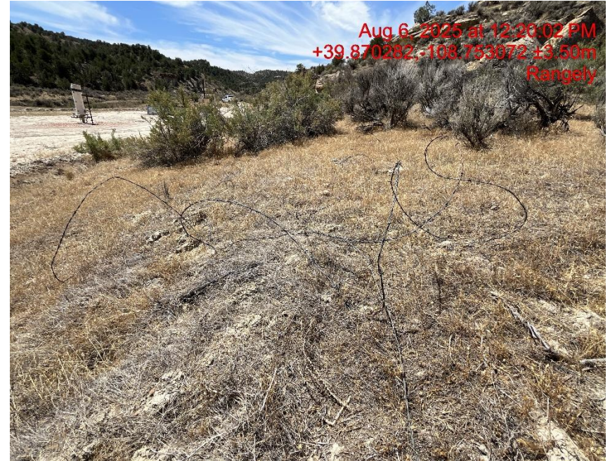
Photo # 1437 Loose barbed wire fencing/wildlife hazard
