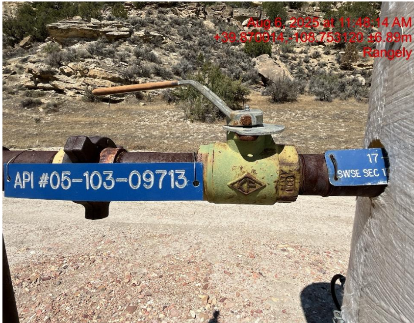
Photo # 1391 Wellhead sign lacks required information
