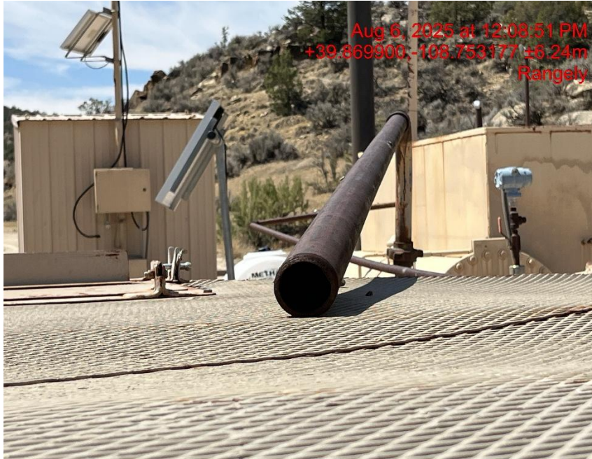
Photo # 1422 Open ended piping/wildlife hazard/available for entry by wildlife
