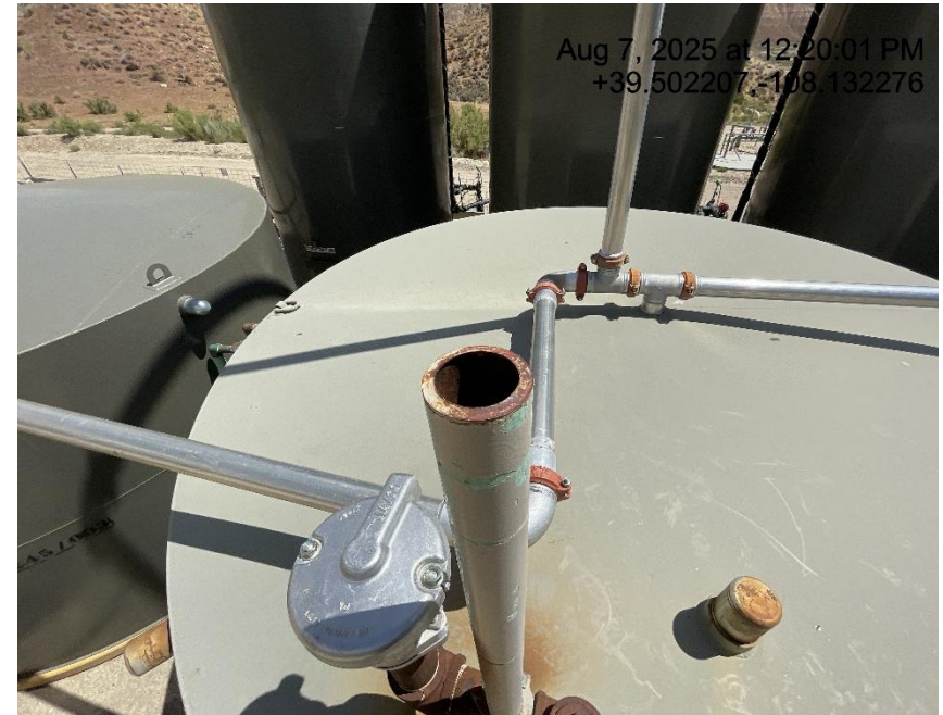
Photo # 9198 Open ended piping on production tank /wildlife hazard
