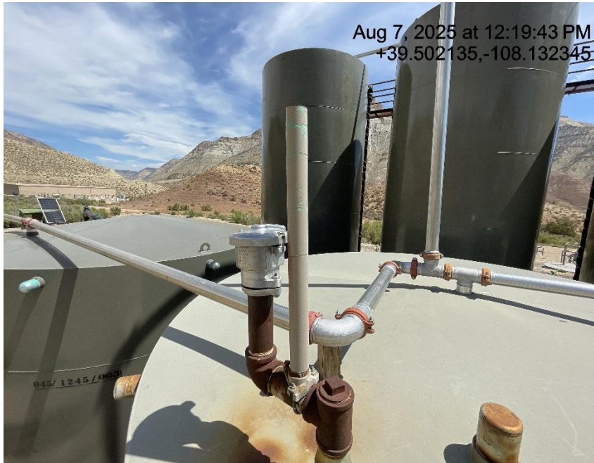
Photo # 9197 Open ended piping on production tank /wildlife hazard
