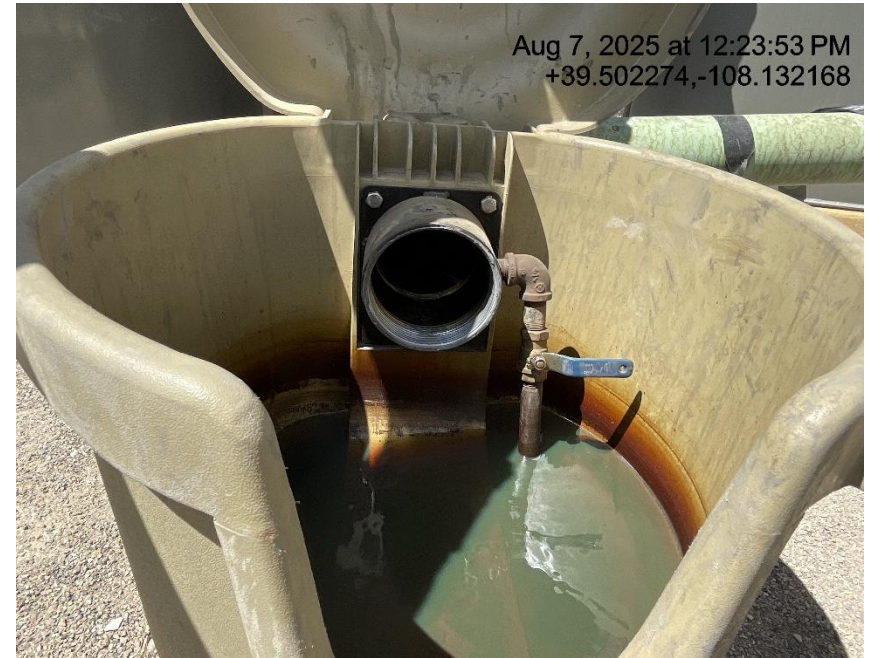
Photo # 9196 Open ended load line
