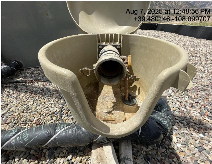
Photo # 9297 Open ended load line
