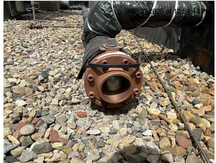
Photo # 9298 Open ended load line
