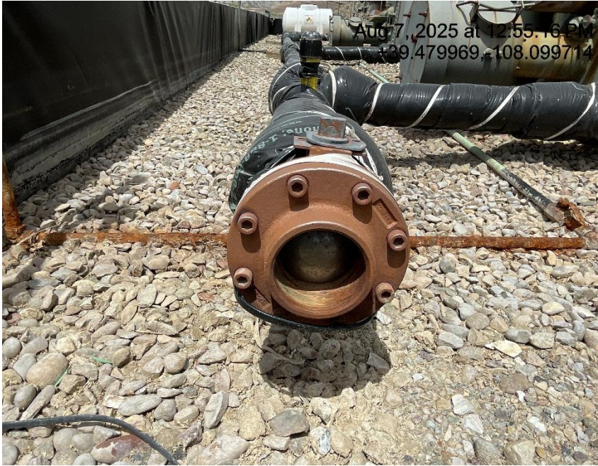
Photo # 9299 Open ended load line
