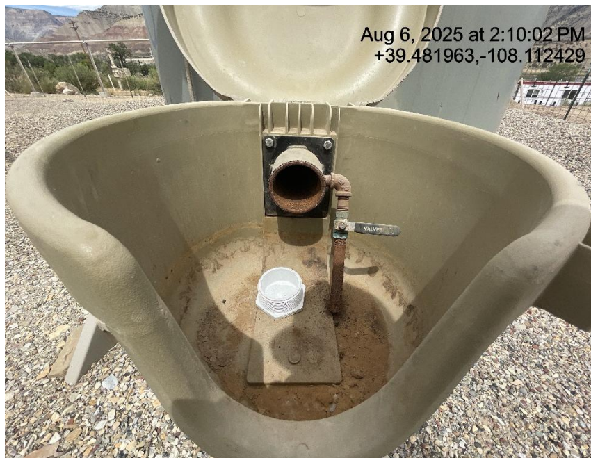
Photo # 8565 Open ended load line
