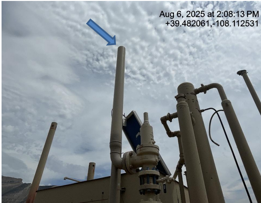
Photo # 8563 PRV vent line does not comply with CECMC pressure safety device rules
