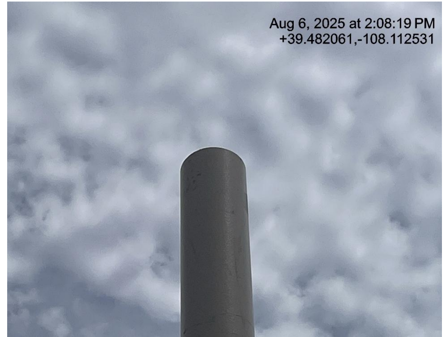
Photo # 8564 PRV vent line does not comply with CECMC pressure safety device rules
