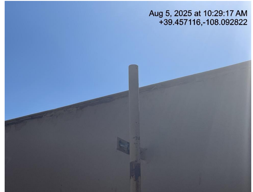
Photo # 7900 PRV vent line does not comply with CECMC pressure safety device rules
