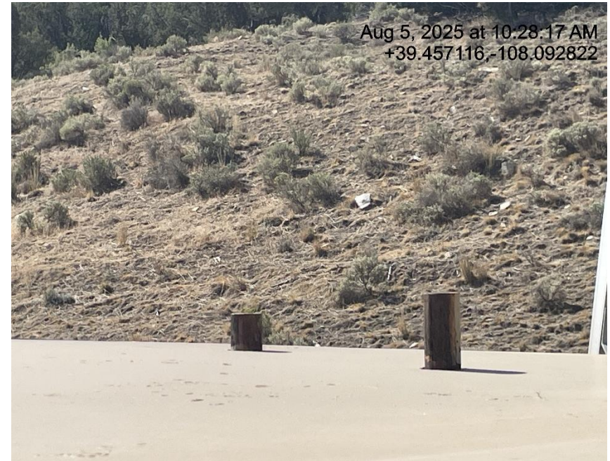
Photo # 7902 PRV & rupture disc vent lines do not comply with CECMC pressure safety device rules
