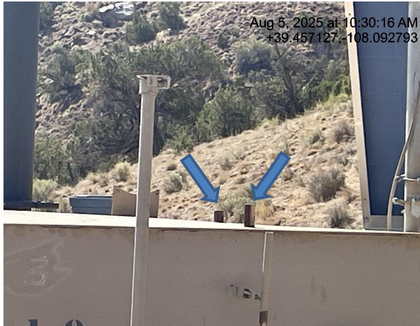
Photo # 7901 PRV & rupture disc vent lines do not comply with CECMC pressure safety device rules
