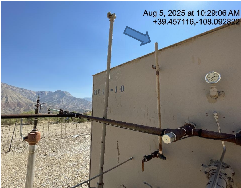
Photo # 7899 PRV vent line does not comply with CECMC pressure safety device rules
