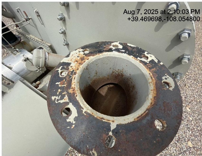
Photo # 9462 Burner exhaust open ended/wildlife hazard /available for entry by wildlife
