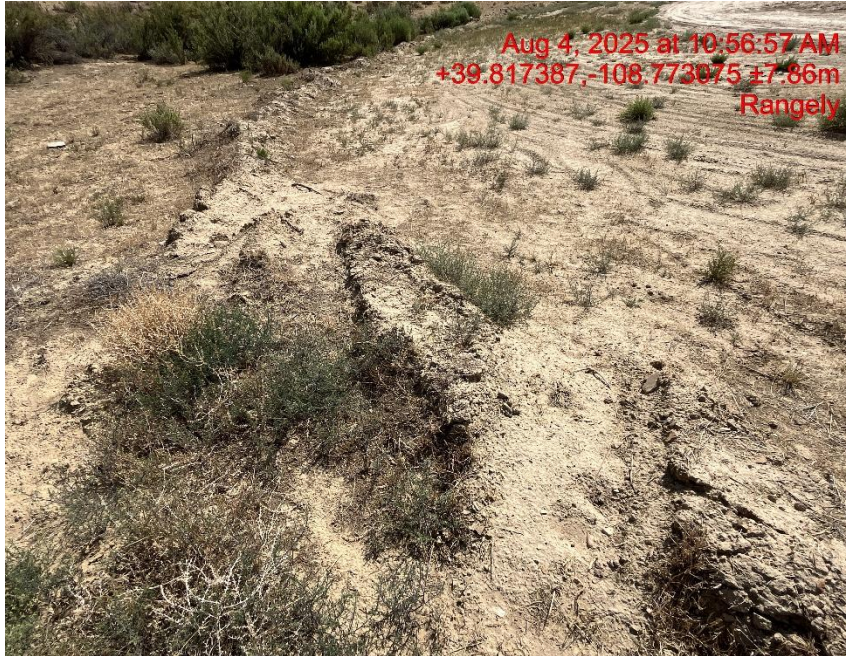
Photo # 1231 Berms on location need maintenance
