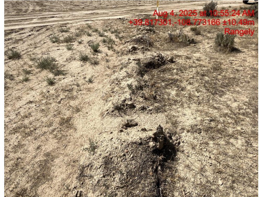
Photo # 1229 Berms on location need maintenance
