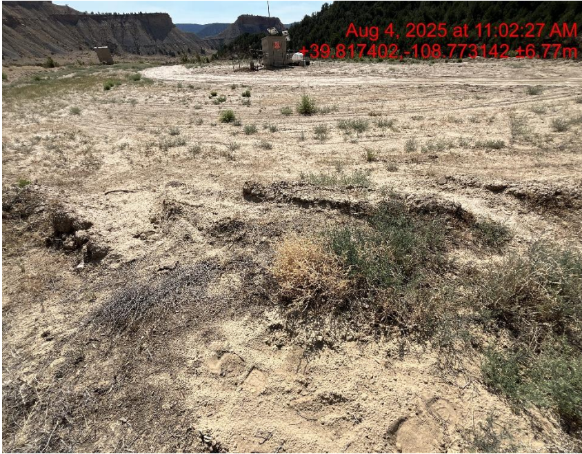
Photo # 1238 Berms on location need maintenance
