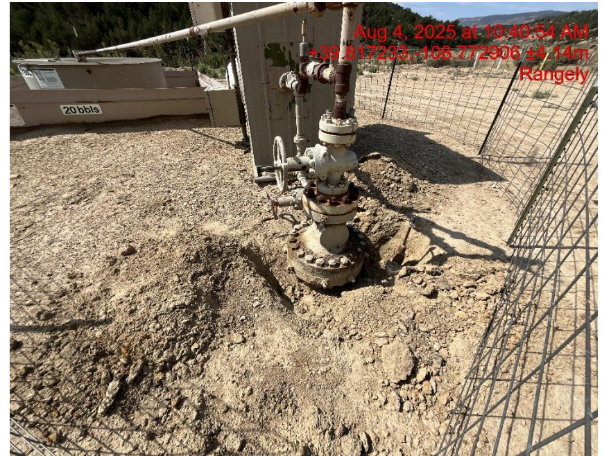
Photo # 1215 Stockpiled soils with no BMP's
