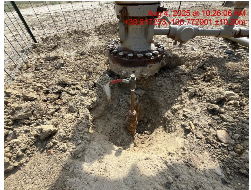
Photo # 1200 Open hole near wellhead/wildlife hazard/personnel safety hazard
