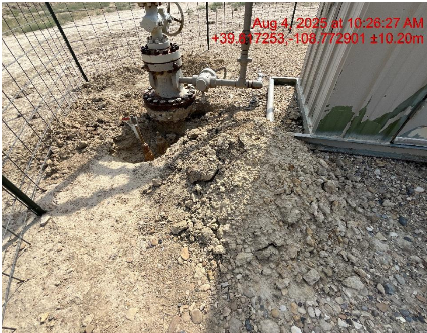
Photo # 1201 Stockpiled soils with no BMP's
