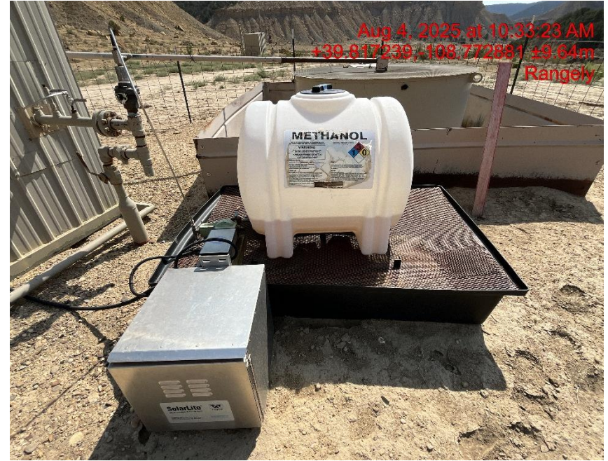
Photo # 1211 Chemical tank label is weathered/not legible
