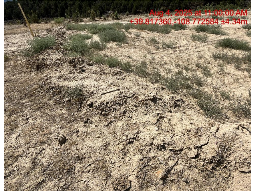
Photo # 1234 Berms on location need maintenance
