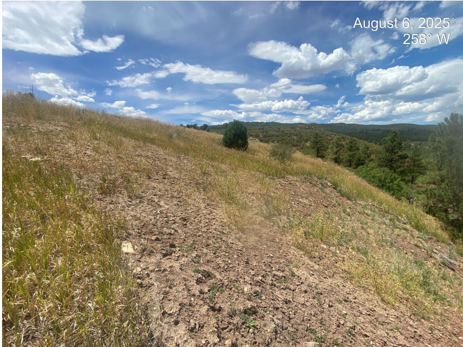
Photo 3. Ground view of collapsed gully erosion and reseeded area.
