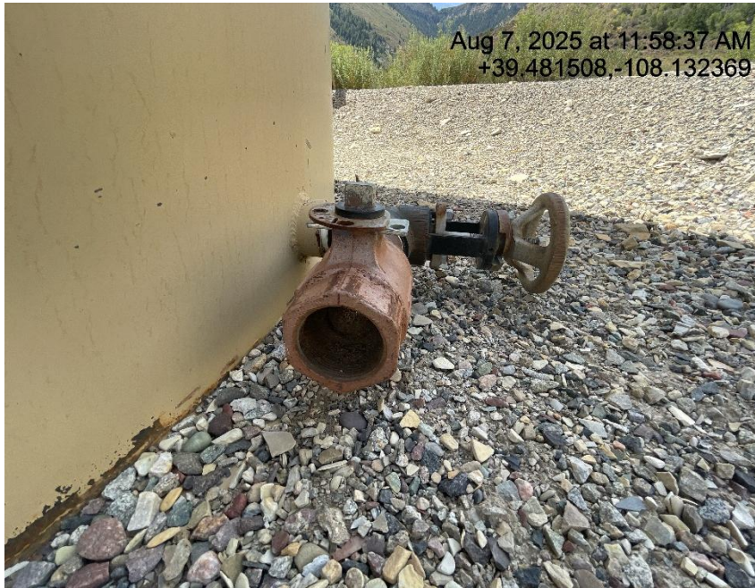
Photo # 9135 Open ended load line
