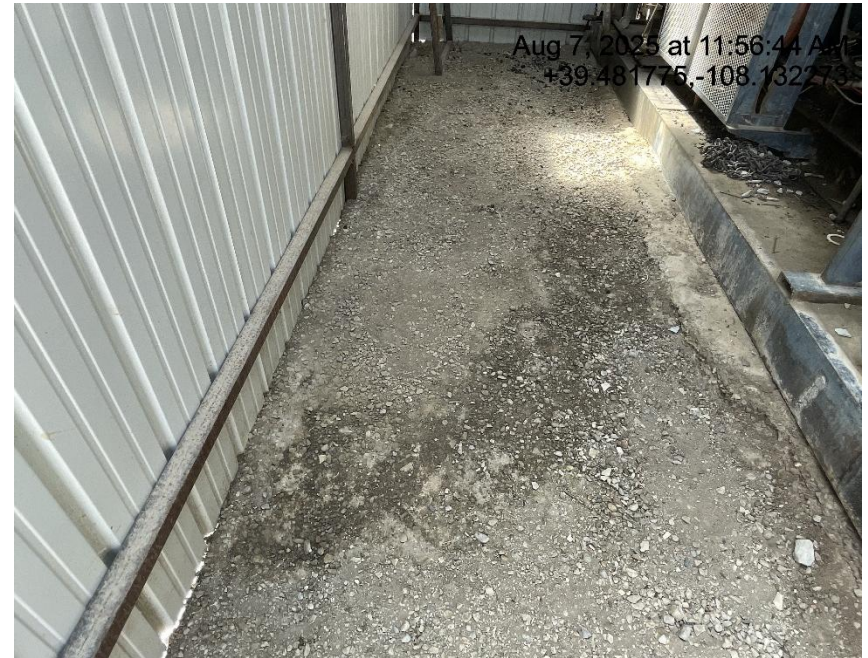
Photo # 9136 Staining near compressor
