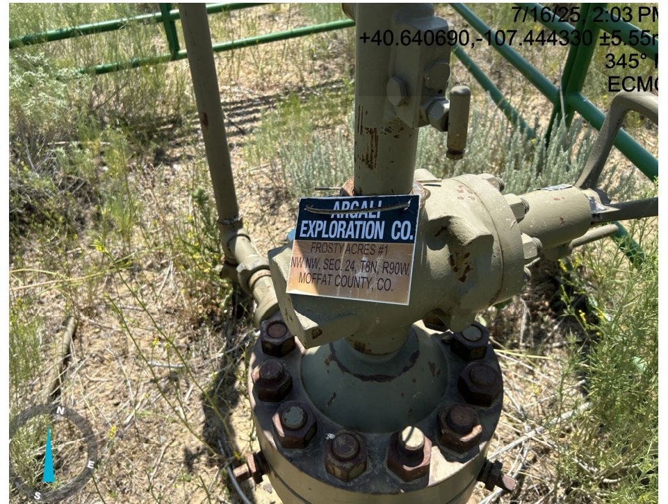
Well signage lacks information
