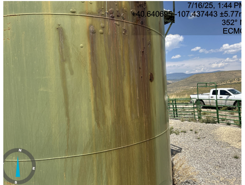
Tank has holes
