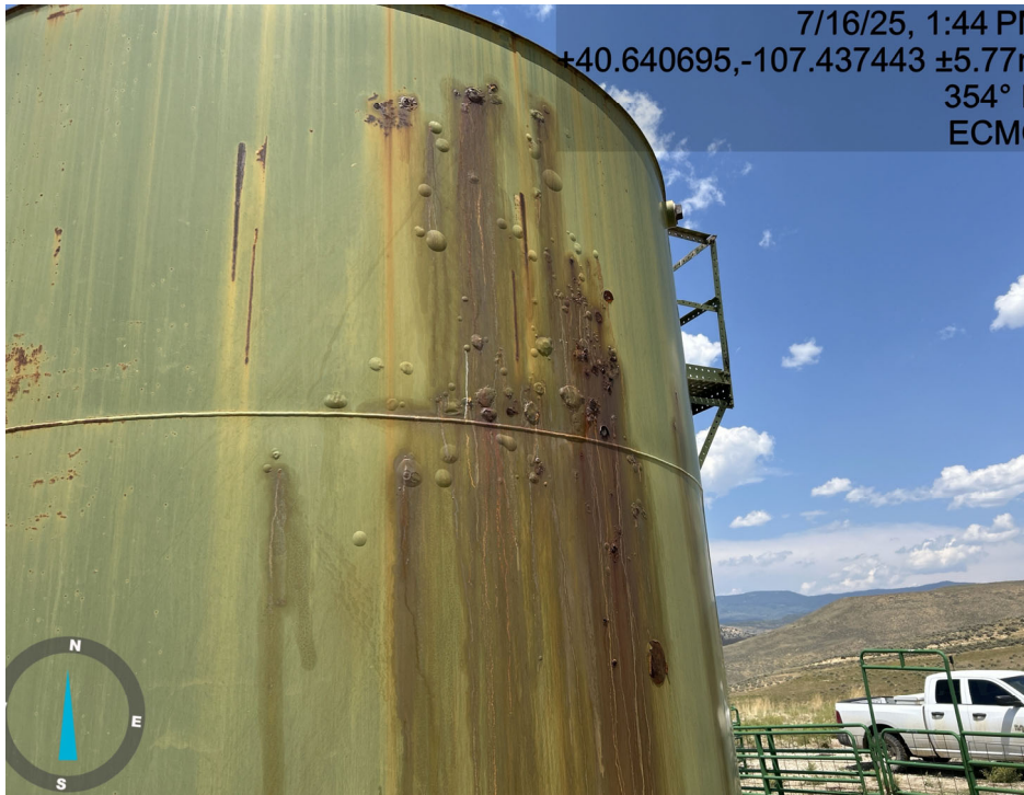
Tank has holes
