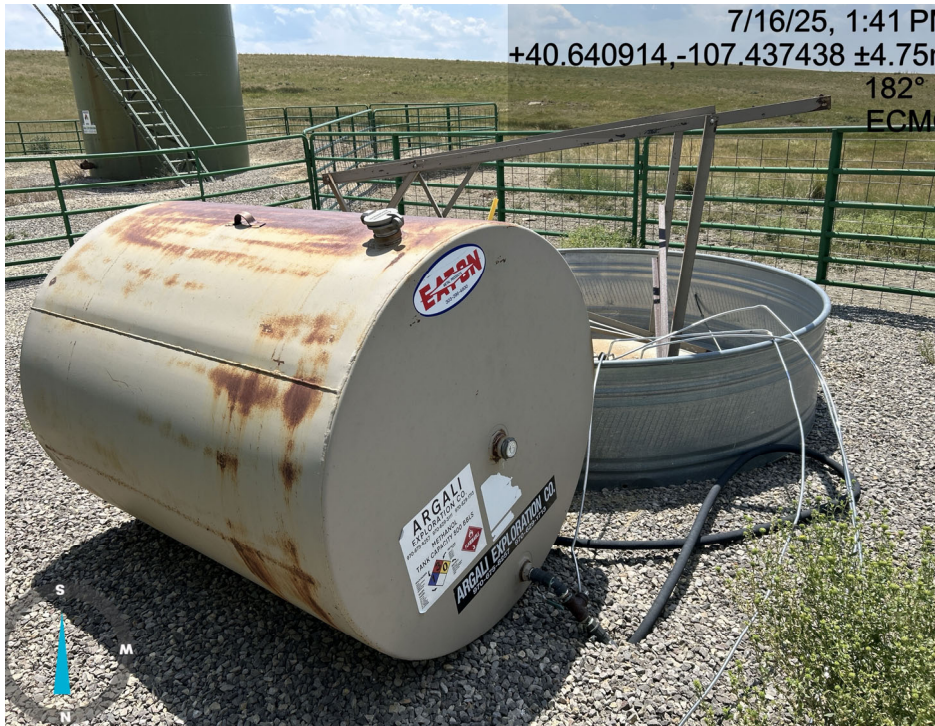
Unused and not contained tank
