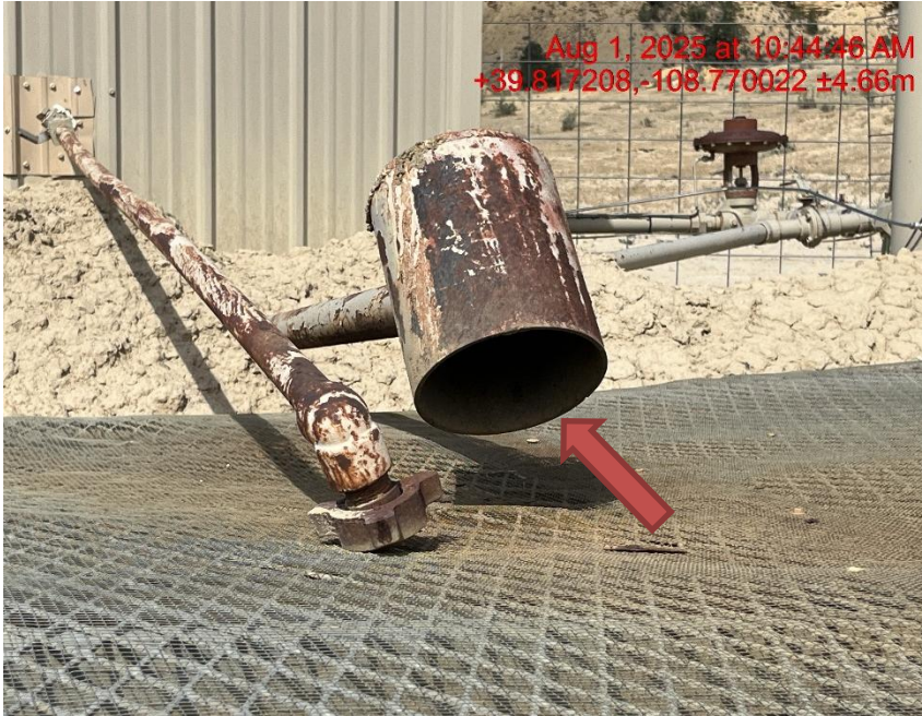
Photo # 1166 Open ended piping/wildlife hazard/available for entry by wildlife
