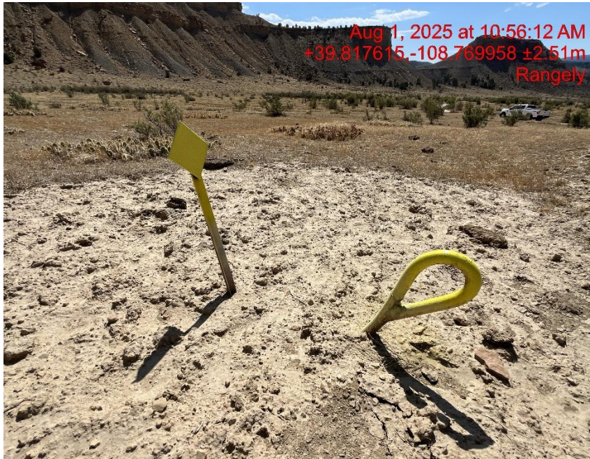
Photo # 1175 Improperly marked deadman
