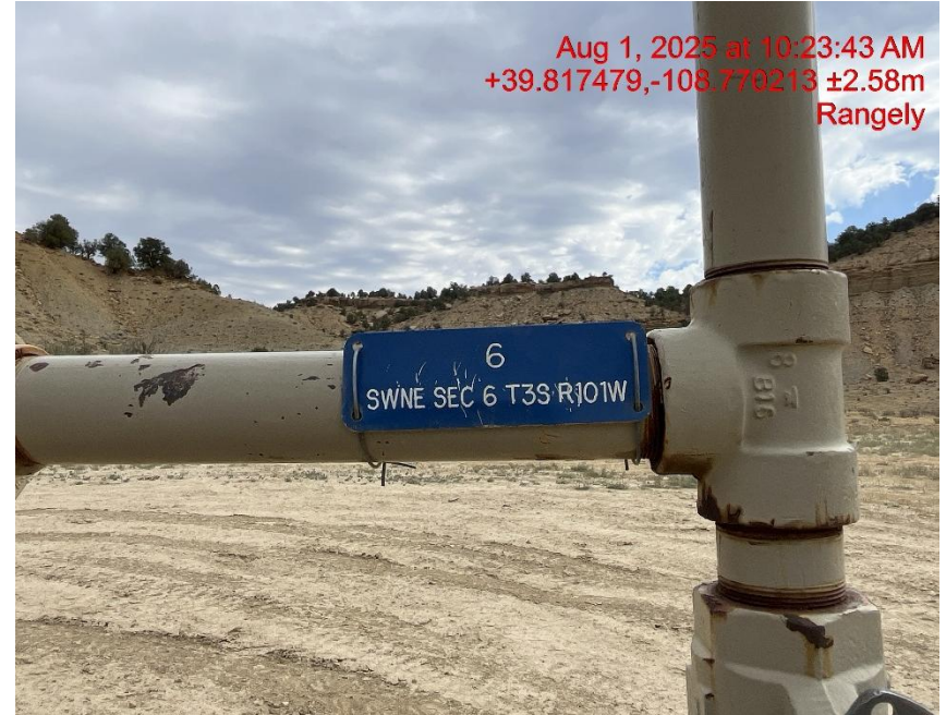
Photo # 1145 Wellhead sign lacks required information
