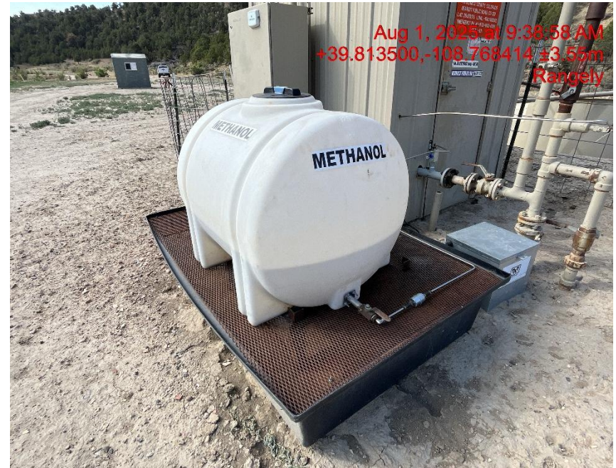
Photo # 1119 Chemical tank lacks required labeling
