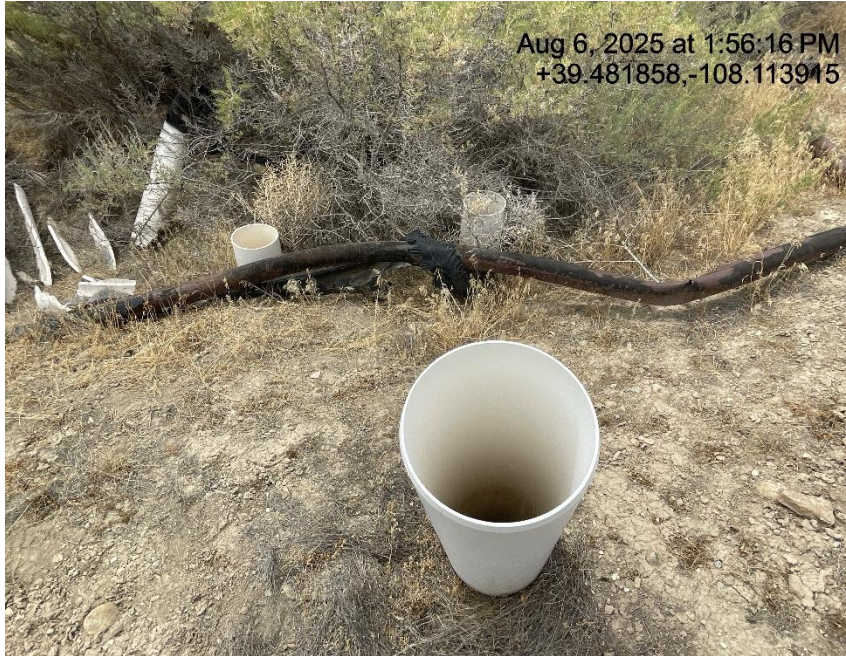
Photo # 8424 Open ended piping/wildlife hazard/available for entry by wildlife
