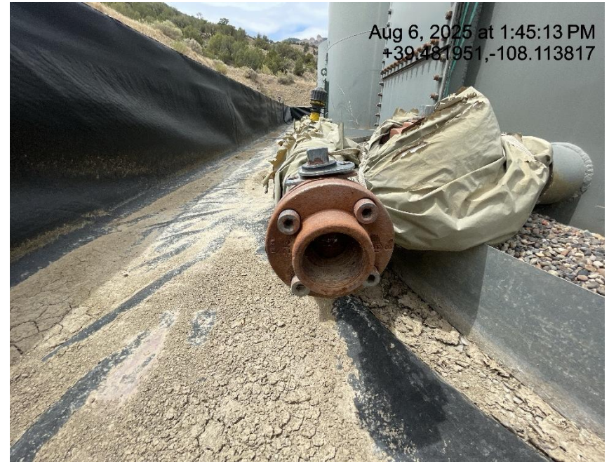
Photo # 8419 Open ended load line
