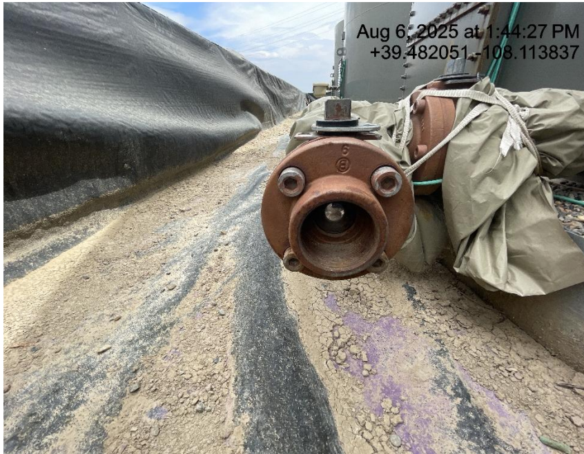
Photo # 8418 Open ended load line
