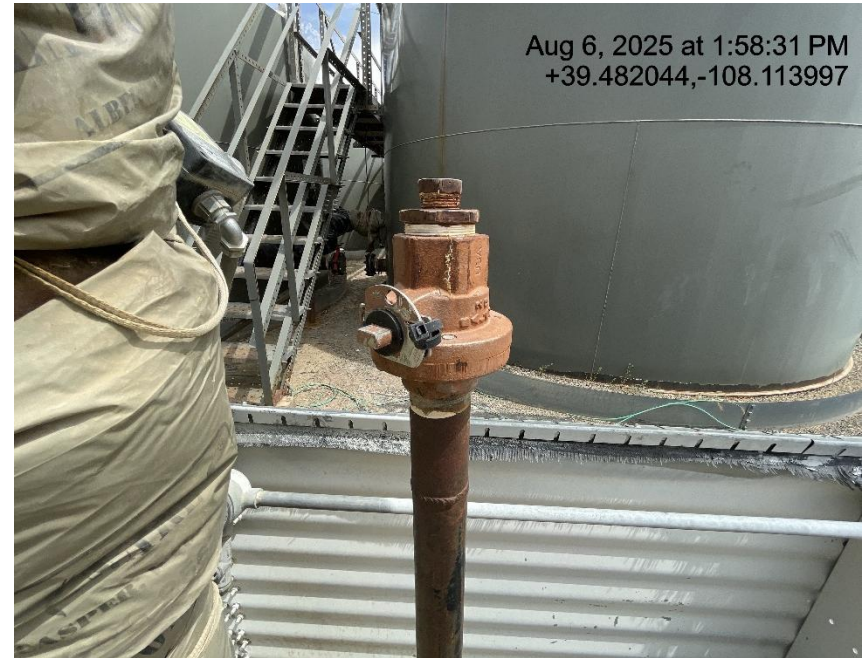
Photo # 8413 Unused flowline lacks lockout tagout (OOSLAT)
