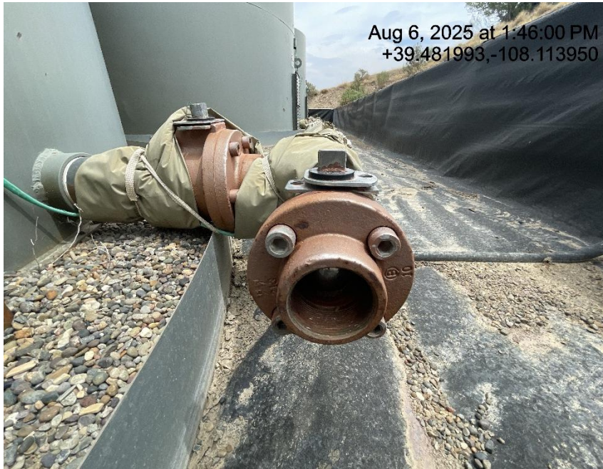
Photo # 8420 Open ended load line
