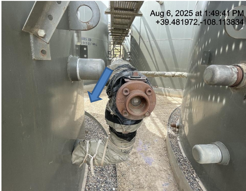
Photo # 8422 Open ended load line
