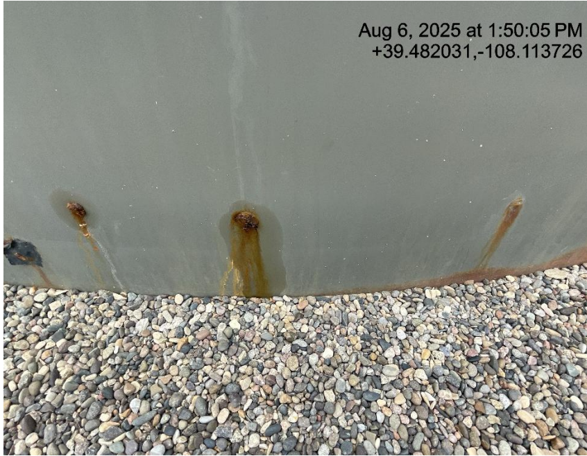
Photo # 8414 Possible tank failure/tank appears to lack integrity
