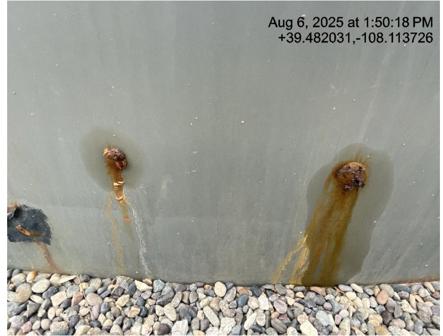
Photo # 8415 Possible tank failure/tank appears to lack integrity
