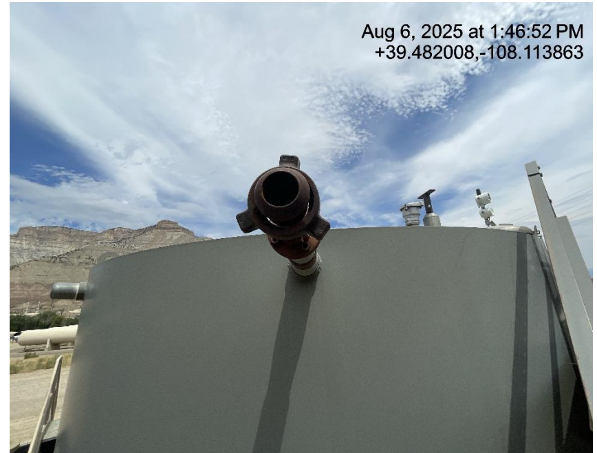
Photo # 8421 Open ended piping/load line
