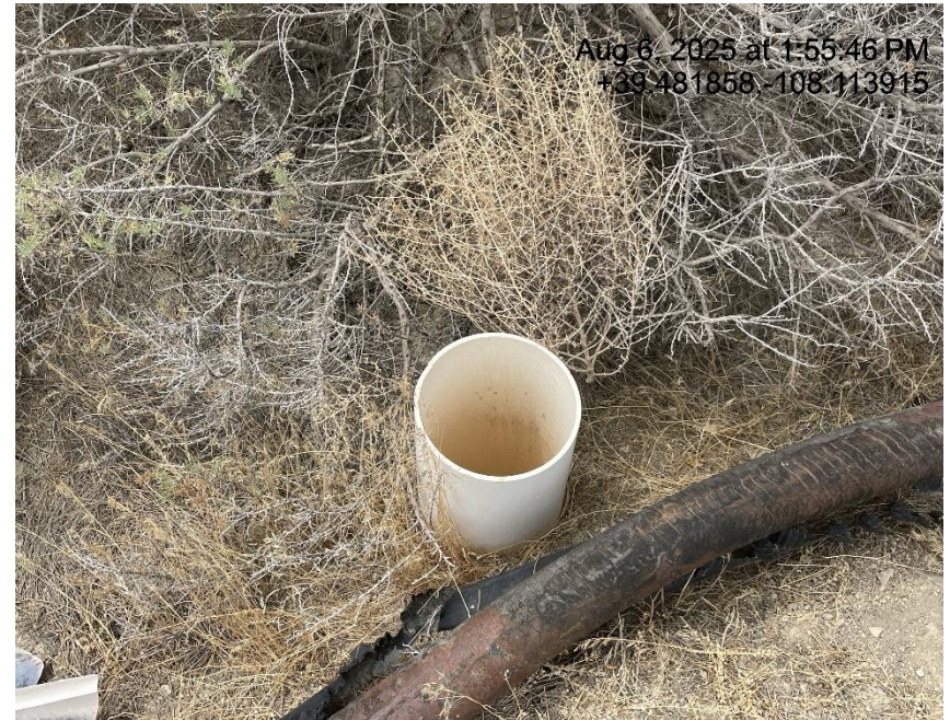
Photo # 8423 Open ended piping/wildlife hazard/available for entry by wildlife
