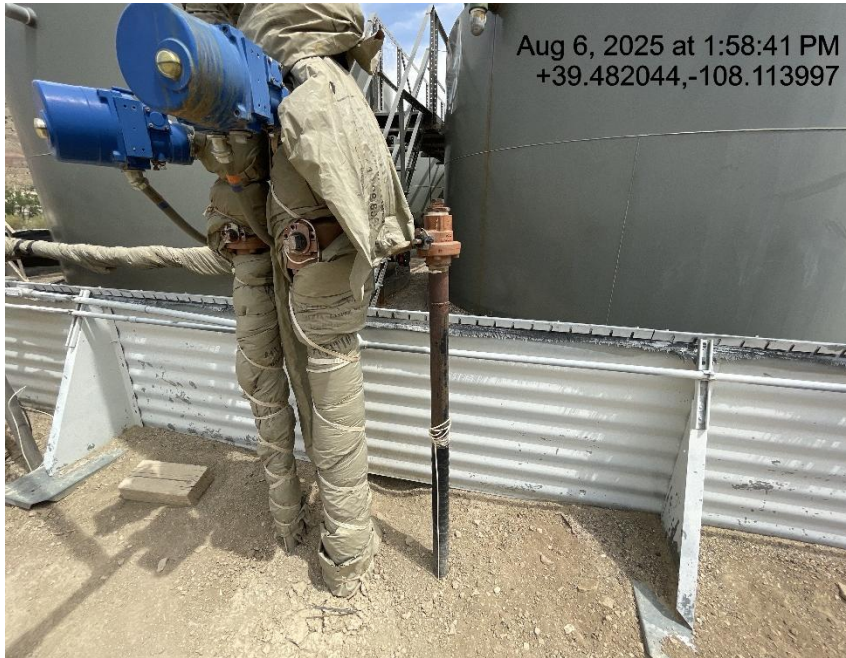
Photo # 8412 Unused flowline lacks lockout tagout (OOSLAT)
