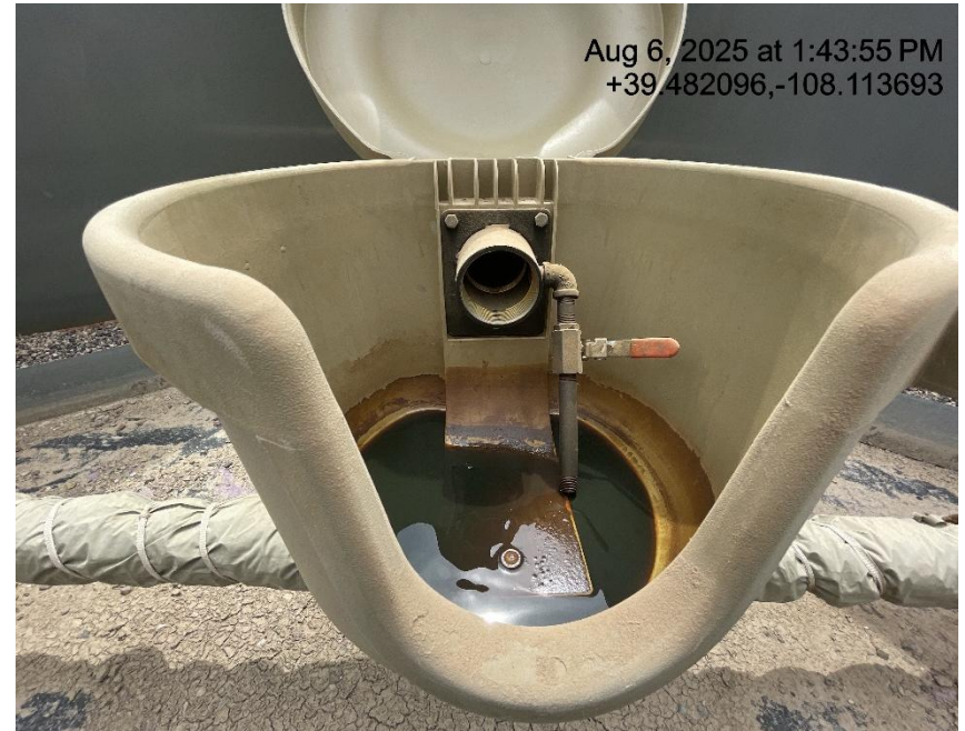
Photo # 8417 Open ended load line
