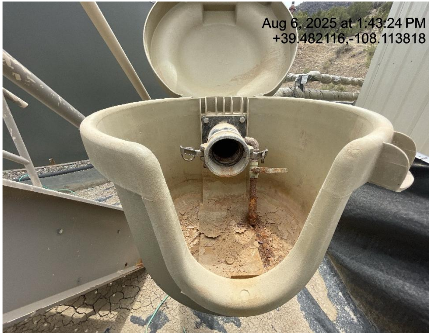
Photo # 8416 Open ended load line
