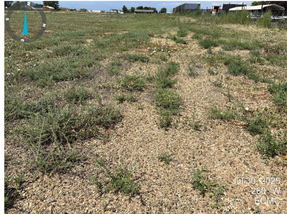
Photo 4. This portion of access road appears to be unused and has a relatively large amount of gravel.
