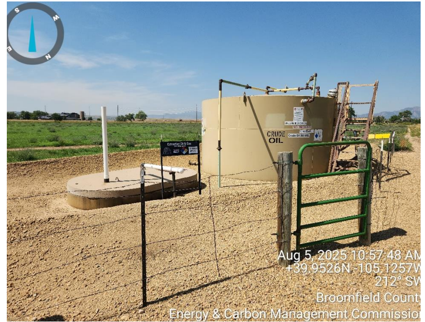
Photo 4 tank battery and equipment
