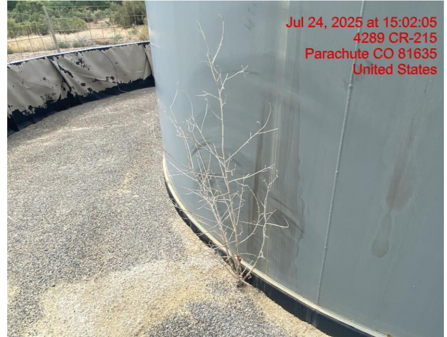
Vegetation Growth Inside Tank Containment – Photo #09959
