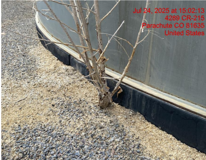
Vegetation Growth Inside Tank Containment – Photo #09960
