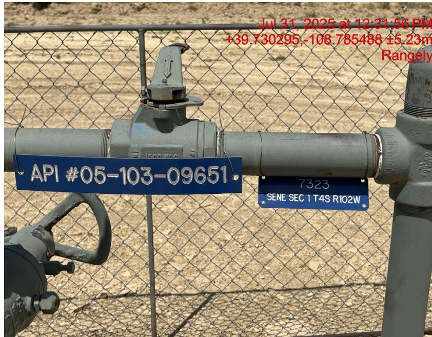
Photo # 1057 Wellhead sign lacks required information
