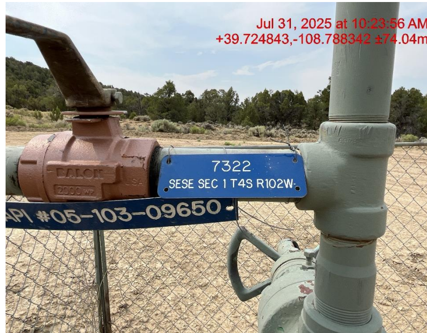
Photo # 1015 Wellhead sign lacks required information
