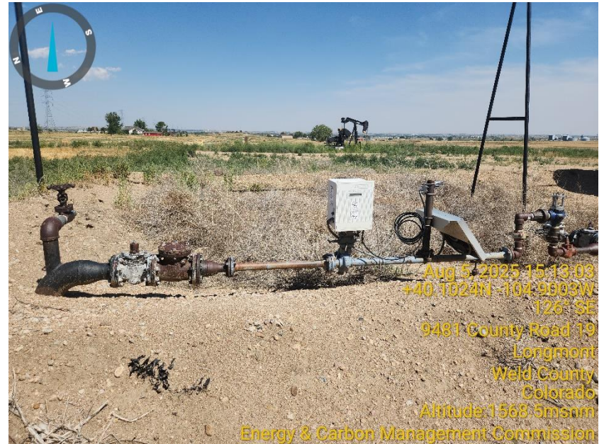
Photo 10 Gas Meter run.
